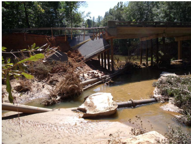
Figure 3-2. Failure of abutment fill in September 2009 Georgia flood accompanied by failure of approach roadway (Hong and Sturm 2010).
