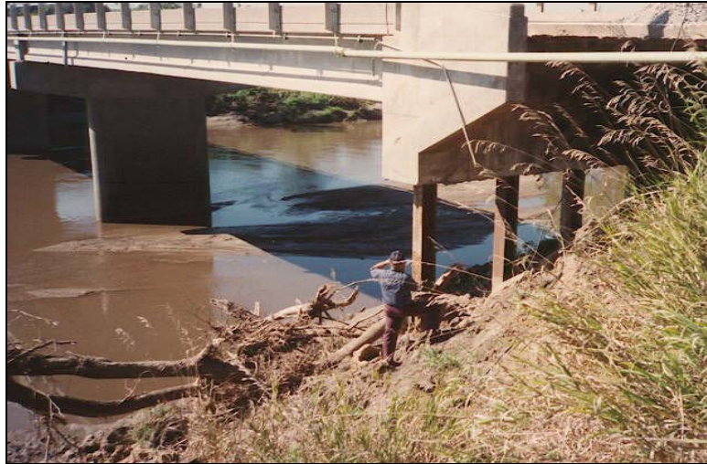
Figure 3-1. A common situation of abutment failure; scour has led to failure and partial washout of the earthfill spill-slope at this abutment. A basic question arises as to how abutment design should take scour into account.
