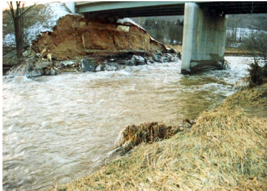
Figure 4-2. Field example of Scour Condition A.
