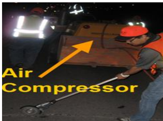
FIGURE 8: NDOR road maintenance air compressor
