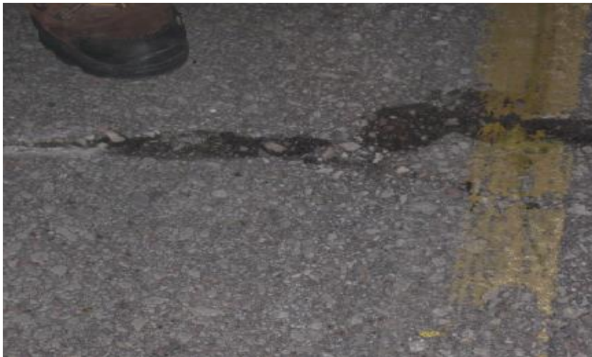
FIGURE 10: Moisture introduced to the pavement from the air compressor.
