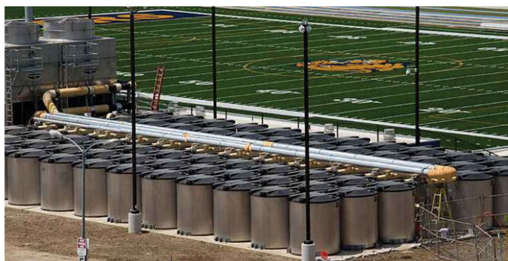
FIGURE H.10 Ice storage system at Southwest College. SOURCE: Courtesy of the Los Angeles Community College District.
