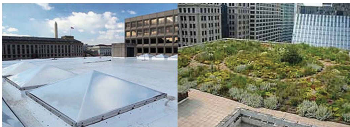
FIGURE 3.5 White roof installed on the headquarters building of the Department of Energy; green roof installed on Chicago's city hall.
