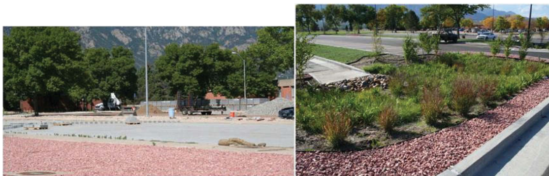
FIGURE E.4 (Left) Permeable Paver Project and (right) bioretention/stormwater management. SOURCE: Courtesy of the U.S. Army.
