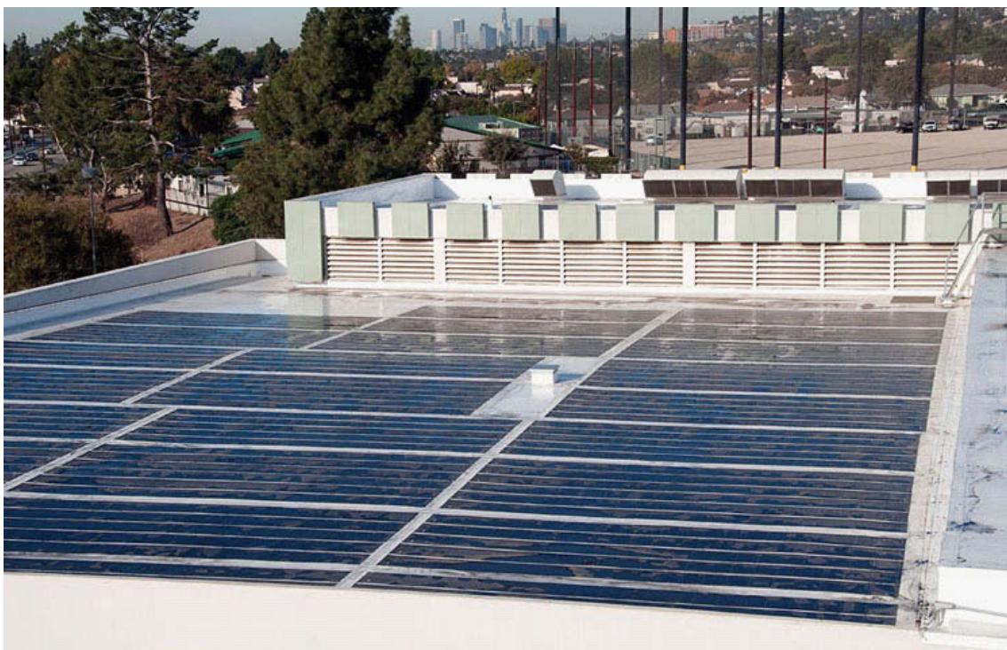
FIGURE H.8 Thin film solar array at East Los Angeles College. SOURCE: Courtesy of the Los Angeles Community College District.
