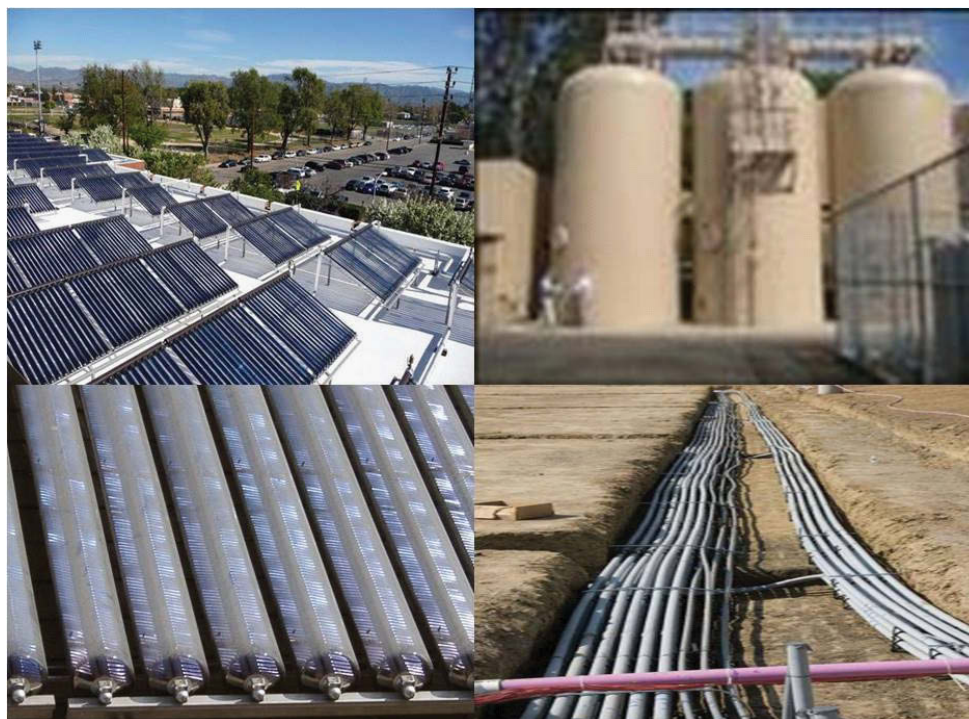
FIGURE 4.6 Valley College central plant components: Solar array ( top left ), hot water storage ( top right ), new infrastructure for delivering power; and vacuum tube heat-pipe collectors ( bottom ). SOURCE: Courtesy of the LACCD.
