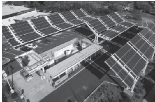
Sacramento Municipal Utility District (SMUD) and BP operate a small demonstration hydrogen refueling station near the SMUD headquarters building.
