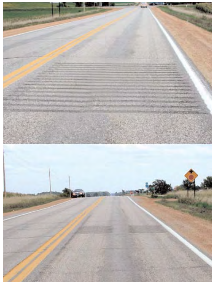
Figure 45. In-lane intersection approach rumble strips (59).
