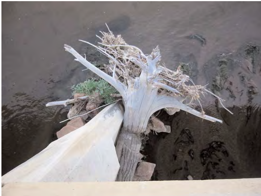
Figure D.11. Looking down on Pier 2 and debris.
