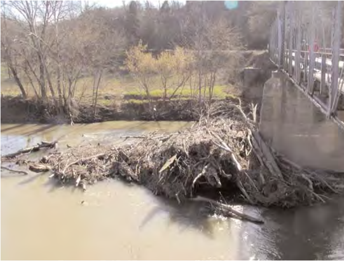
Figure 3.21. Collapsed triangular debris pile with conical profile geometry.
