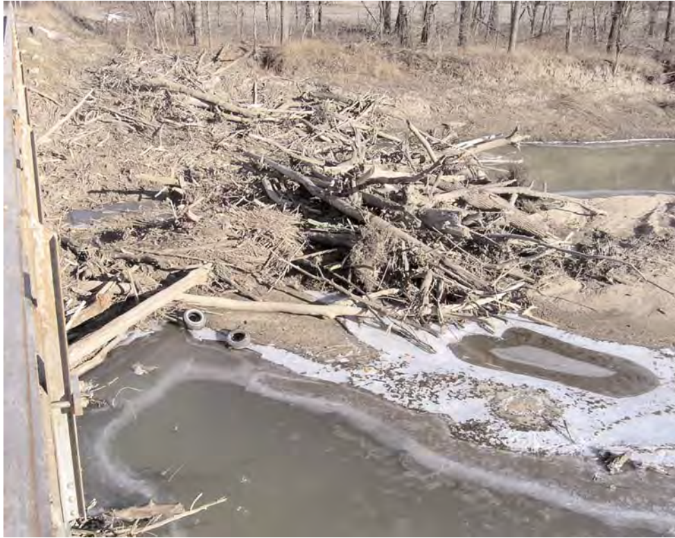
Figure 3.26. Collapsed debris pile with an inverted cone geometry.
