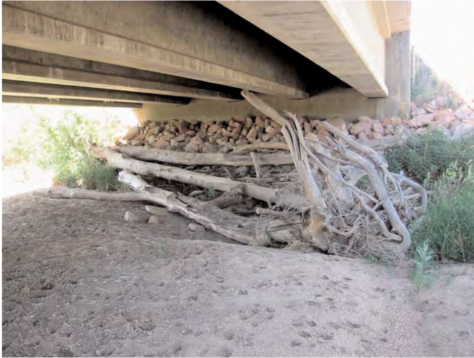
Figure D.12. Debris on right abutment.
