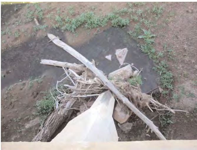
Figure 3.13. View looking down at debris cluster and scour hole on the upstream end of Pier 1 of Bridge WEL 50/67A.
