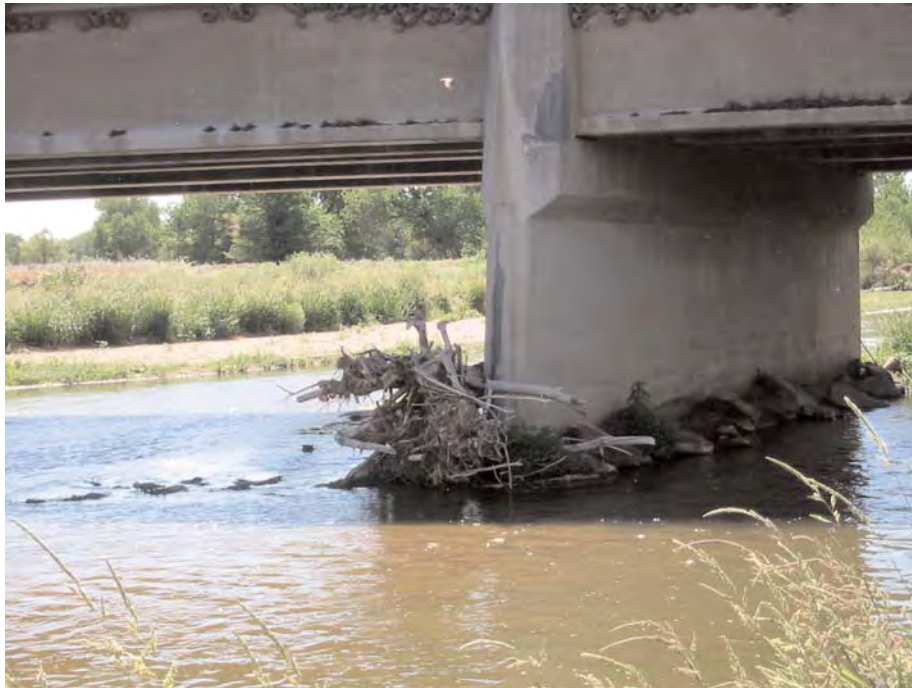
Figure D.10. Pier 2 with debris.
