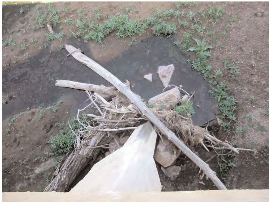
Figure D.9. Pier 1 with debris and scour hole.
