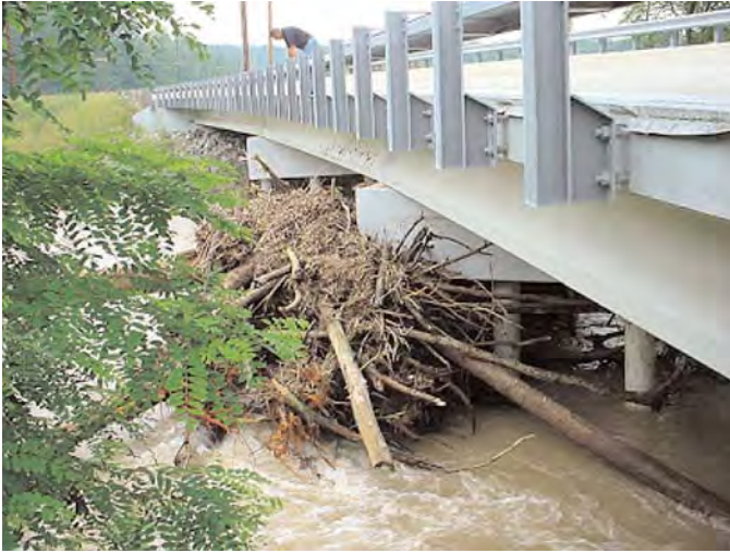
Figure 3.86. A fully developed debris mass creates significant scour potential.
