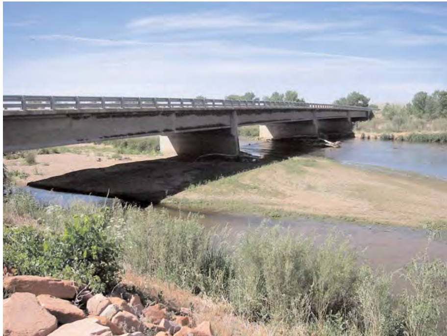
Figure D.7. Looking upstream left bank to right bank at Bridge RD-50.
