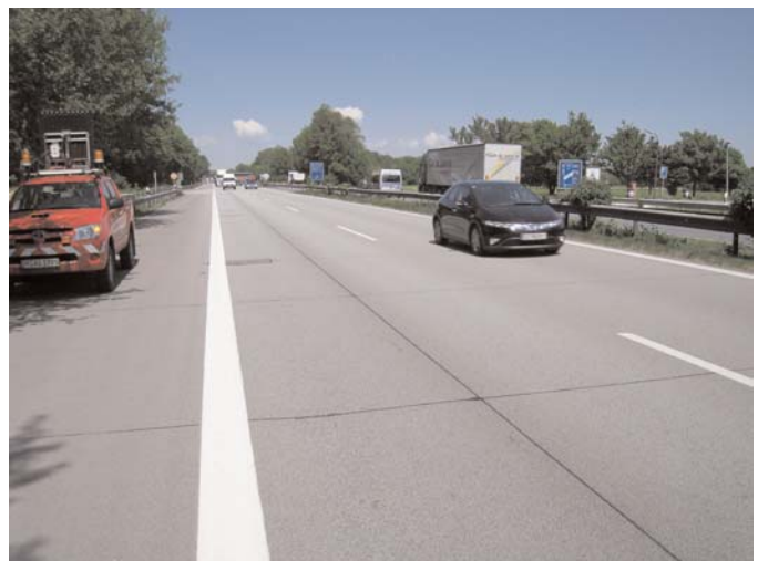
Figure 4.14. A93 motorway in Germany showing SMA over JPCP with sawed and sealed joints after 13 years of heavy truck traffic.
