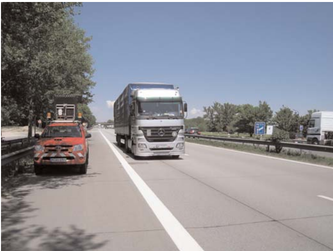
Figure 4.16. A93 SMA/JPCP motorway near Munich, with sawed and sealed longitudinal and transverse joints.
