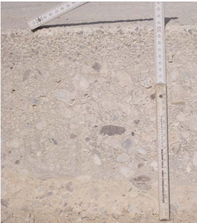
Figure 3.13. Cross-section of completed two-layer PCC pavement. Smaller aggregates are in the top layer, and larger aggregates are in the lower layer.
