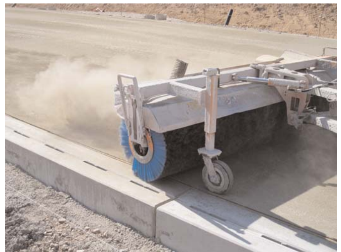
Figure 3.17. Top: Brush operator conducts more hand brushing tests at regular intervals to determine when to initiate second pass with brush. Bottom: Final of two passes with brush to complete EAC texture.
