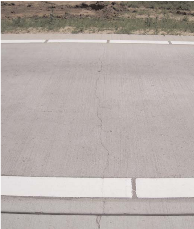
Figure 4.9. Transverse cracking on the unsurfaced A73 CRCP.
