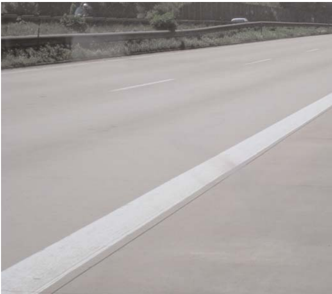
Figure 3.2. Loss of texture, especially noticeable in wheelpaths, in longitudinal burlap drag textured sections along A93 motorway (km 1.490–1.910) near Kiefersfelden, Germany.
