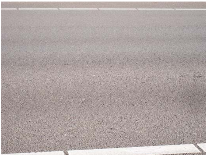
Figure 4.2. Raveling of porous AC surfacing in the outer lane wheelpaths of the A12 motorway.
