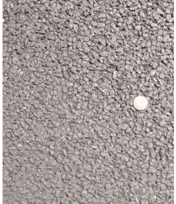
Figure 4.6. Double-layer porous AC surface of the A73 motorway, recently opened to traffic.
