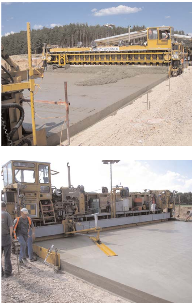
Figure 3.9. Front (top) and rear (bottom) views of the second paving machine, responsible for the upper of two PCC layers. Note the use of a super-smoother at the rear of the machine.
