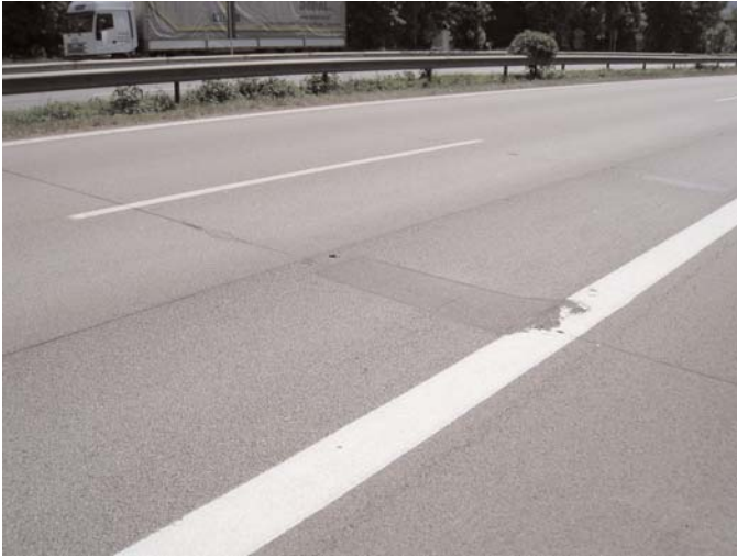
Figure 4.15. A93 SMA over JPCP with sawed and sealed transverse and longitudinal joints. Note patch placed in wheelpath of transverse joints.
