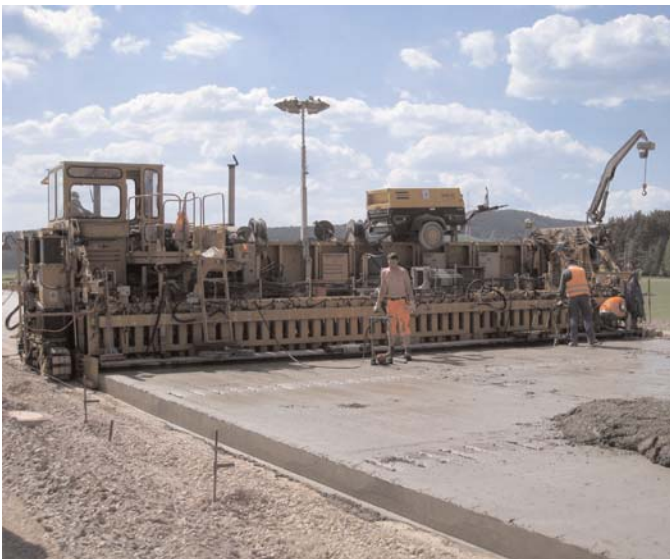
Figure 3.7. Front (top) and rear (bottom) views of the first paving machine, responsible for the lower of two PCC layers.
