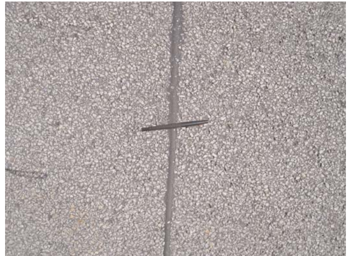
Figure 4.18. Close-up of A93 SMA surface and transverse sawed and sealed joint over JPCP after 13 years of heavy traffic. Some transverse joints required patching for unknown reasons.
