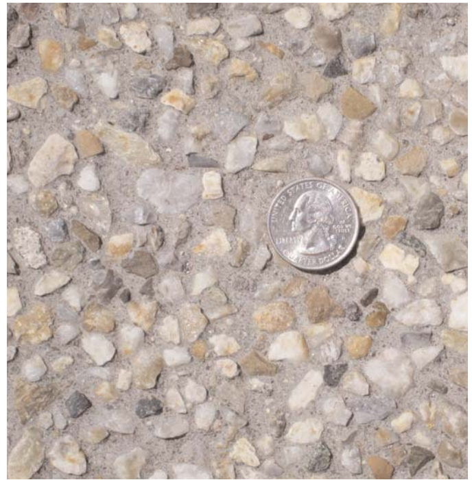
Figure 3.44. Exposed aggregate texture on the Vorchdorf section reveals top-layer use of crushed gravel with a maximum aggregate size of 11 mm.
