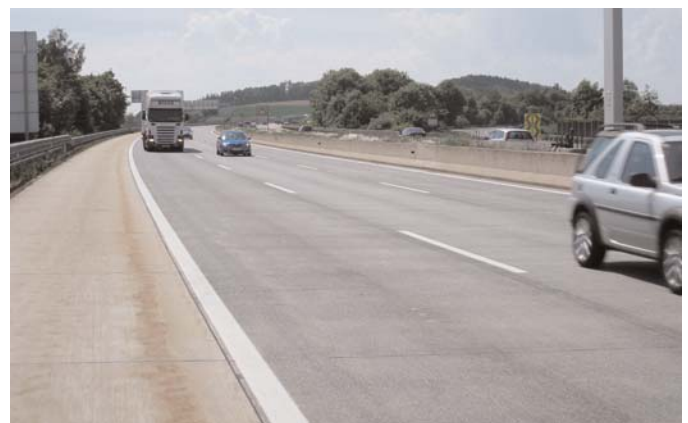
Figure 3.45. View of the Traun section along A1. Note the lack of texture on the shoulder.
