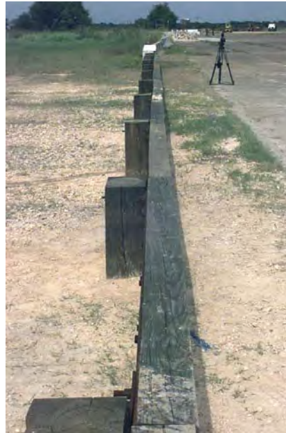
Figure 11. Type B Steel-Backed Timber Guardrail System.
