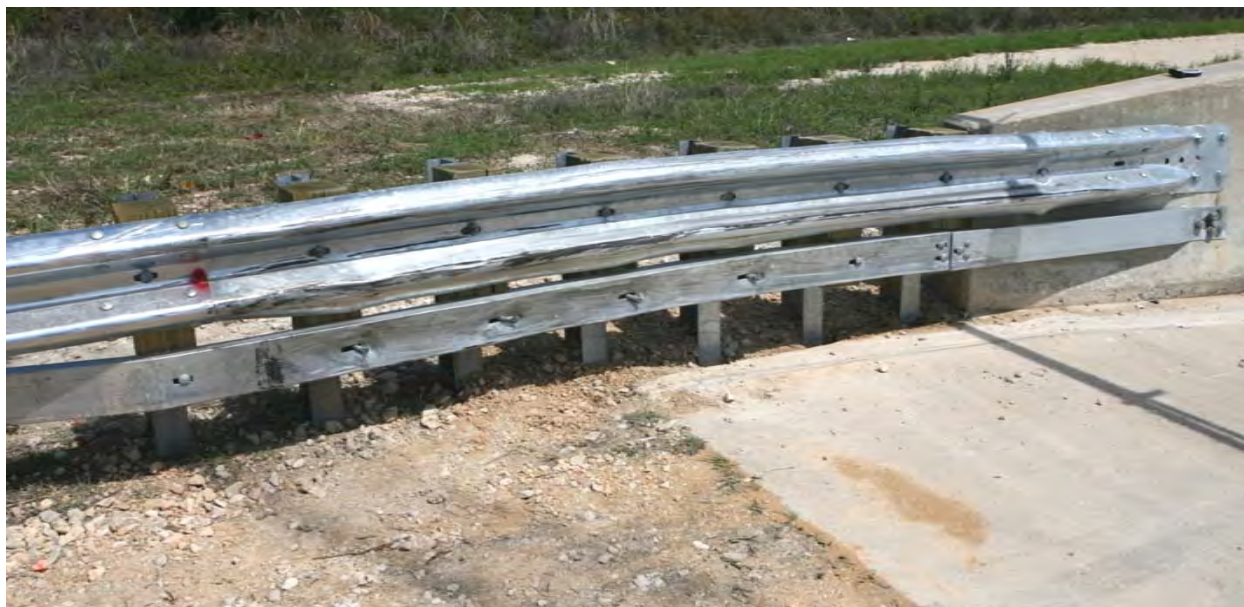
Figure 61. PennDOT W-Beam Transition after MASH Test 3-21.
