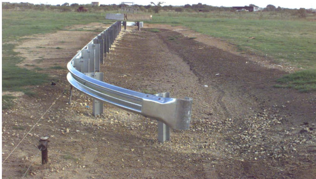
Figure 27. Vermont Low-Speed Guardrail Terminal.
