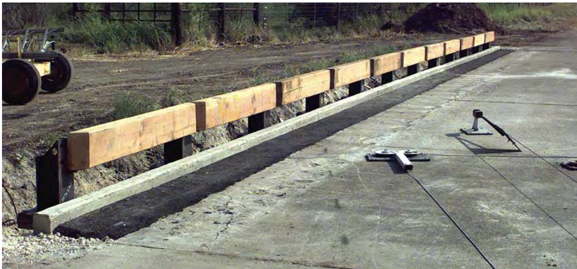
Figure 14. Glacier Park Removable Timber Guardrail System.
