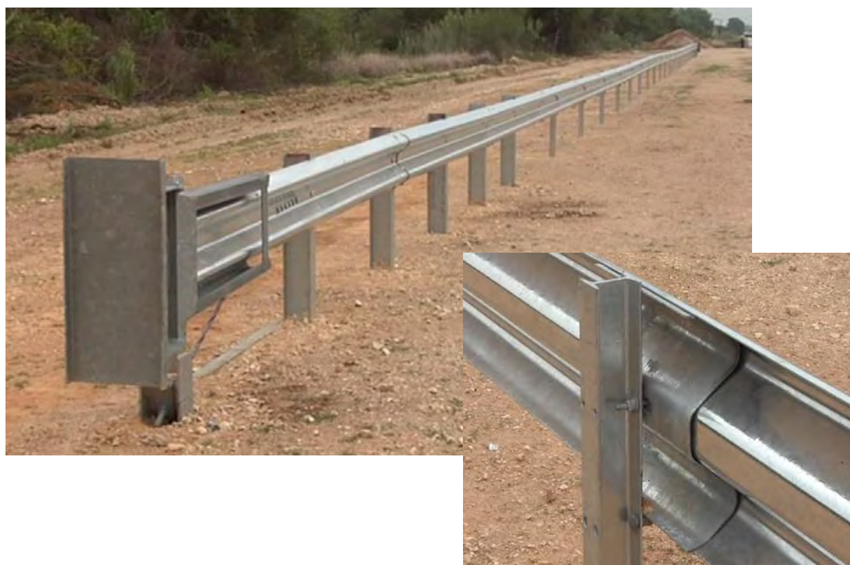
Figure 78. Modified G2 Weak Post W-Beam Guardrail prior to Testing.
