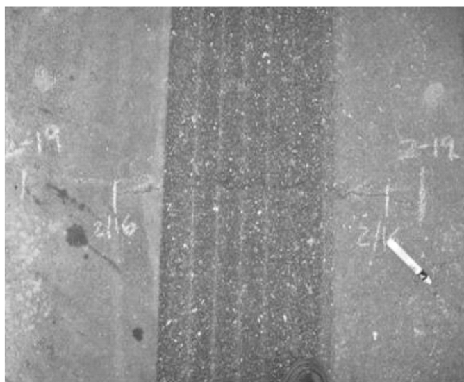
Figure 2-19. Cracks observed in the aged section
