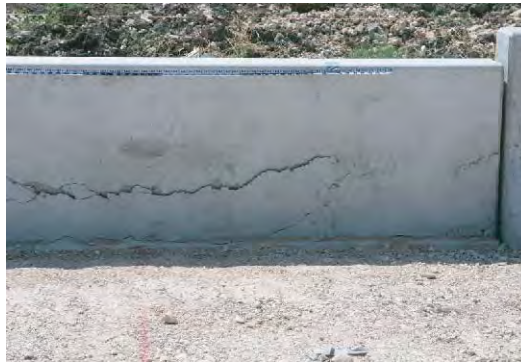
(b) Closeup front view of the barrier
