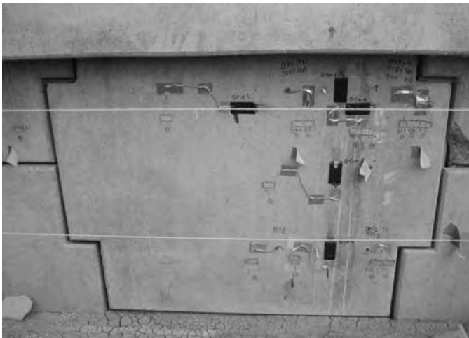
Figure 5.88. Panel surface after test (Test 3).
