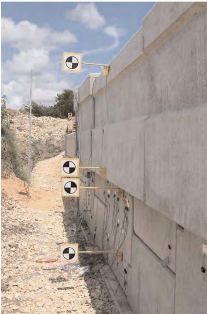
Figure 5.94. Location of displacement bars affixed on the barrier and panels (Test 4).
