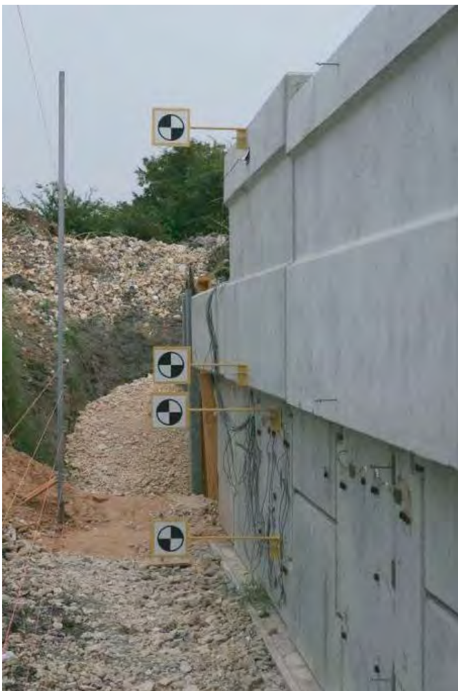
Figure 5.45. Location of displacement bars affixed on the barrier and panels (Test 1).
