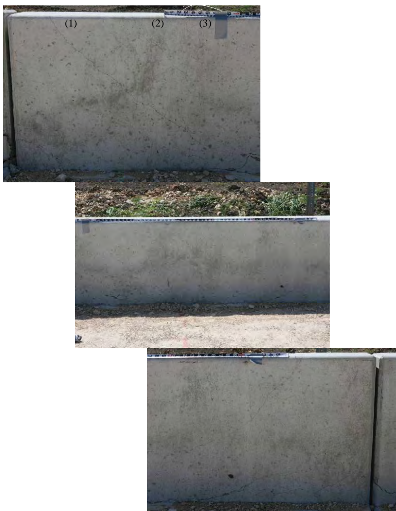
(b) Closeup front view of the barrier
