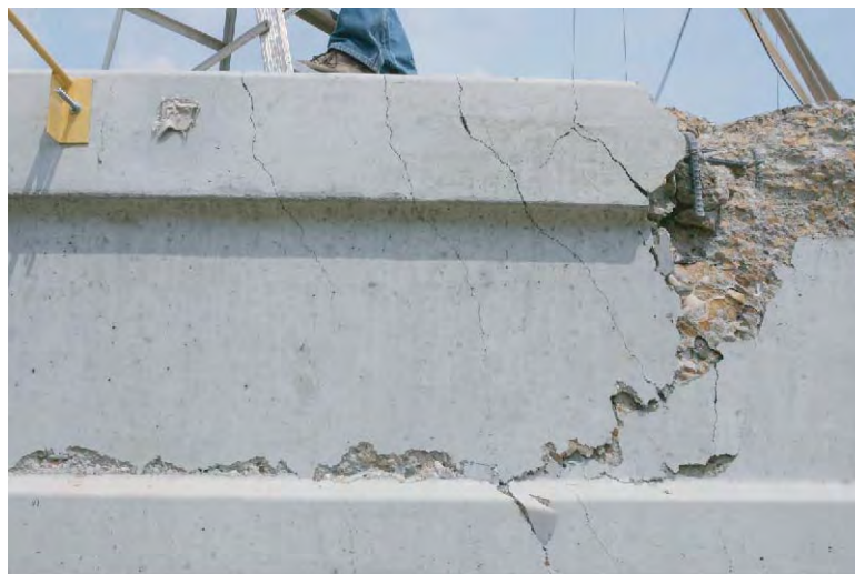
(f) Closeup back view of the barrier
