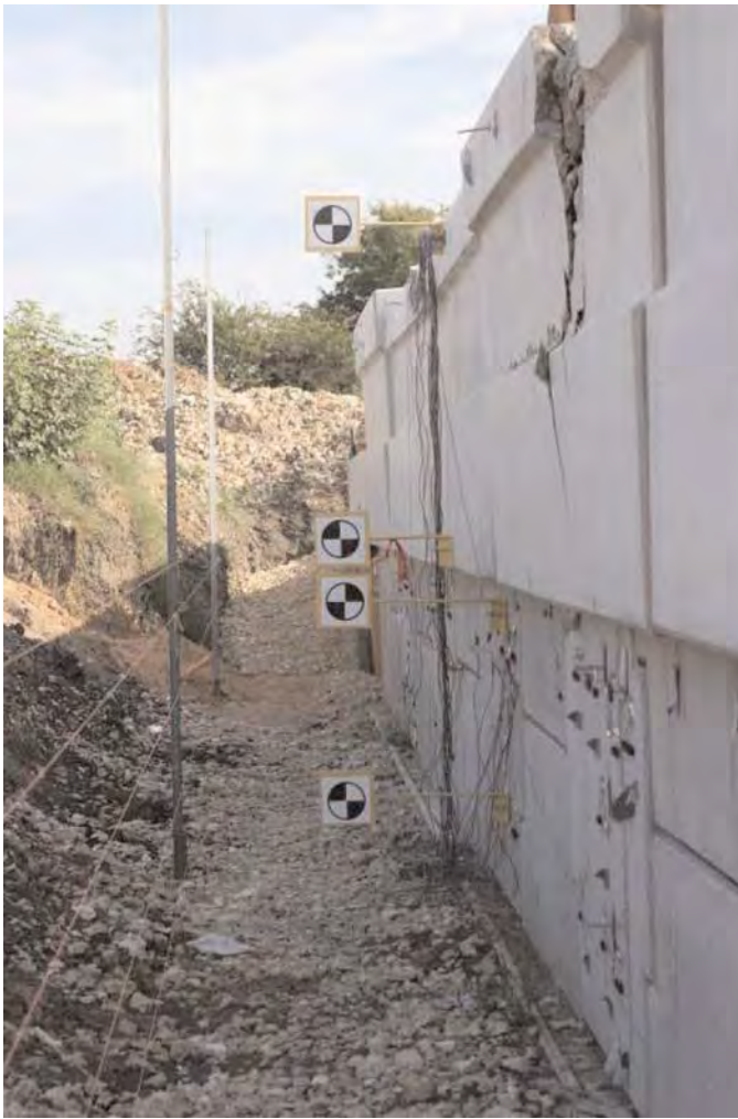
Figure 5.78. Location of displacement bars affixed on the barrier and panels (Test 3).
