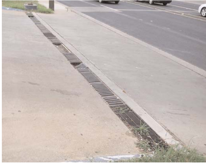
Exhibit 5-80. Damaged grates in driveway need repair.
