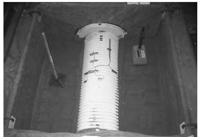
Figure C-57. Photograph taken during backfilling of T4 showing PVC pipe with sand placed above the springline of the pipe; the manual compaction plate and nuclear density gauge are also shown.
