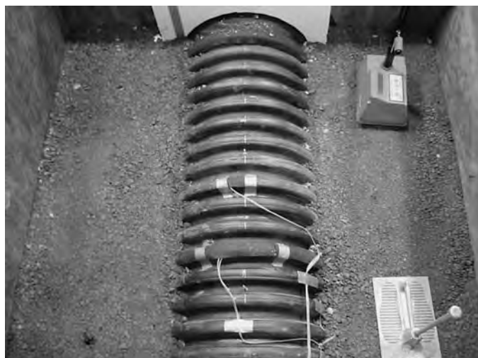
Figure C-58. Photograph taken during backfilling of T5 showing HDPE pipe with granular “A” placed just above the springline of the pipe; the nuclear density gage is also shown.
