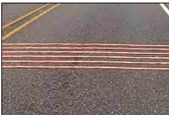
FIGURE 5 Raised transverse in-lane rumble strips.
