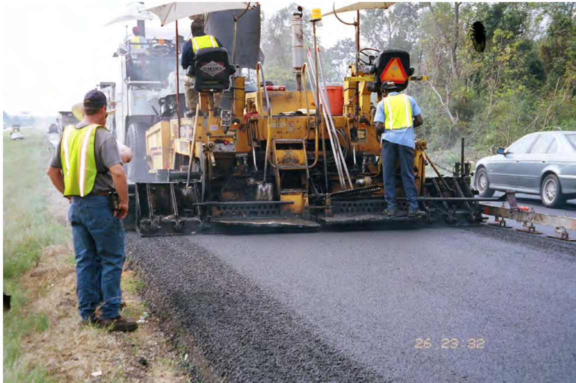
Figure B.6. Placement of the 1.5-inch SMA Overlay Tested During the I-85 Rehabilitation Project Near Auburn, Alabama (refer to Figure B.8)
