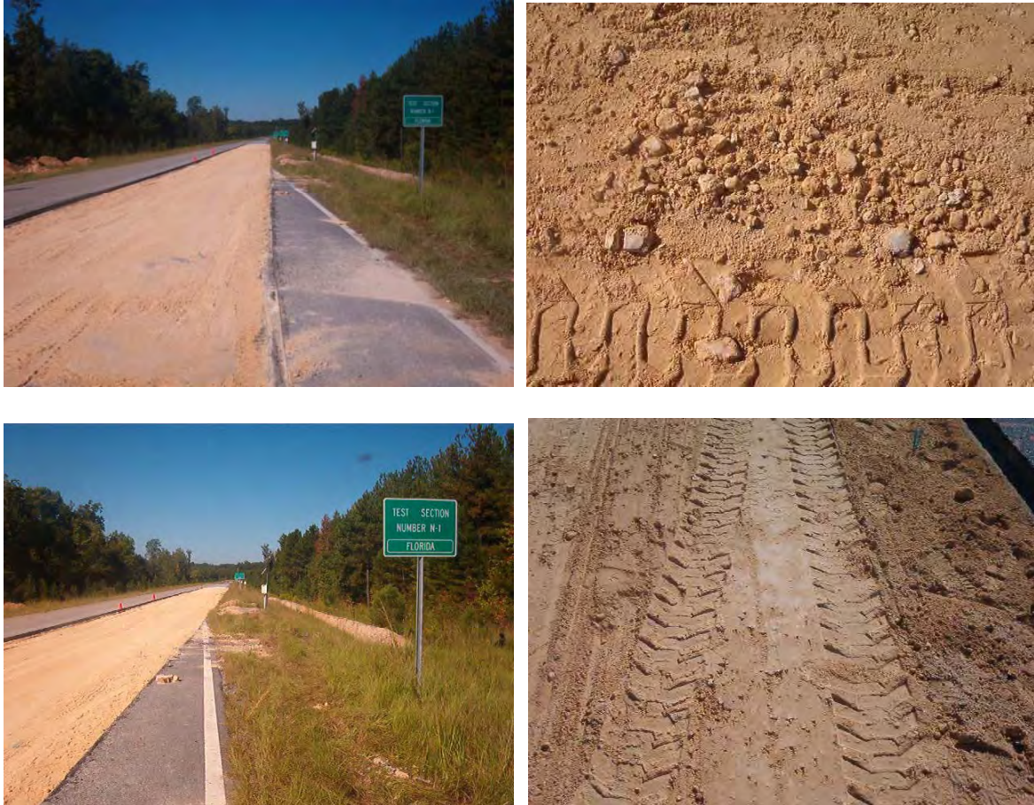
Figure B.65. Florida Limerock Base Placed in NCAT Test Sections N-1 and N-2
