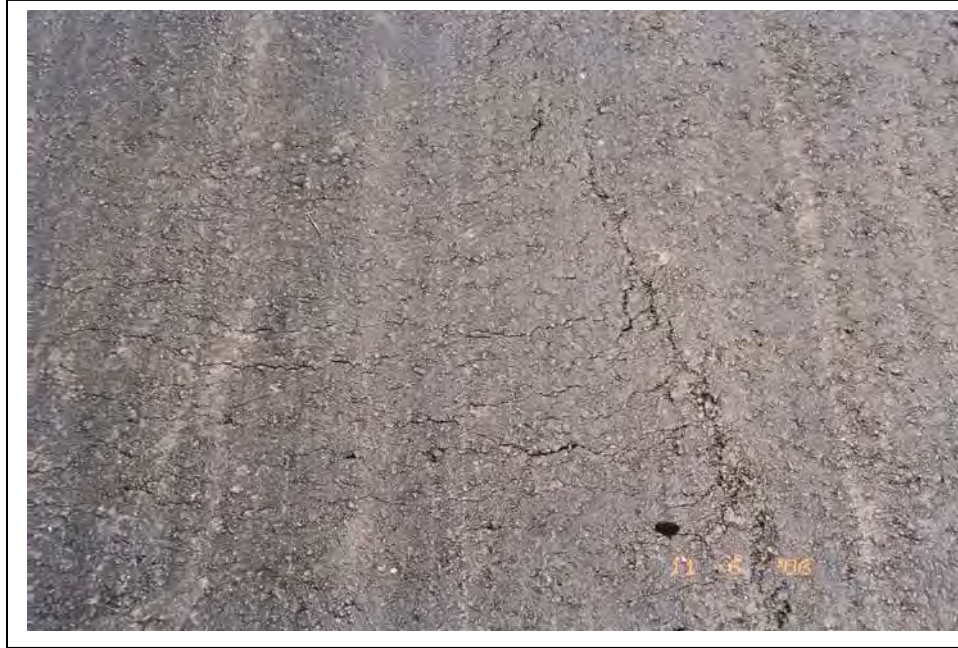
Figure B.75. Checking and Mat Tears Exhibited Along the Florida Section N-1
