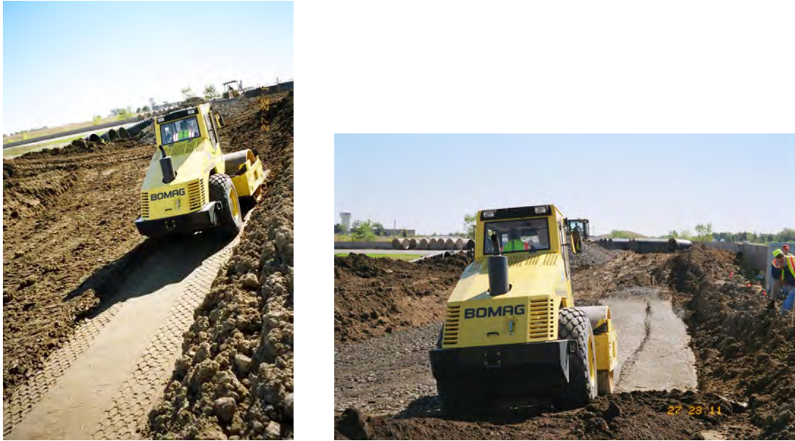
Figure B.2. Embankment Soil at MnROAD Facility Being Compacted with the BOMAG VariControl Device/Roller
