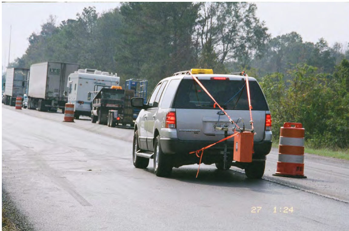
Figure B.7. Compacted SMA Overlay and Ground Penetrating Radar Testing Along the SMA Overlay Project Near Auburn, Alabama (refer to Figure B.8)
