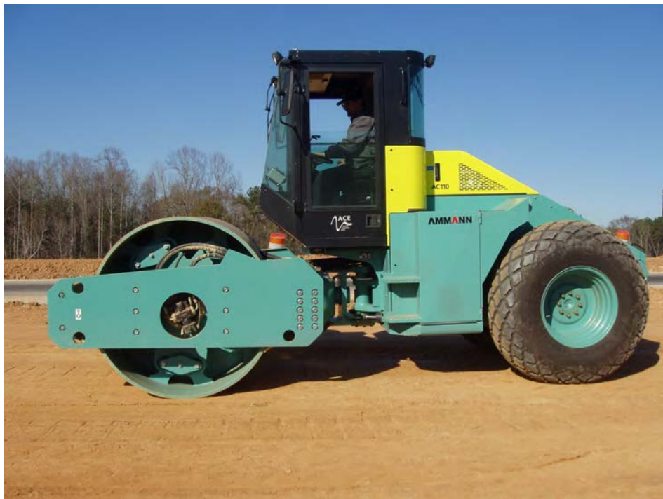
Figure B.18. Intelligent Compaction Roller of the Embankment Soil at Exit 51 Ramp – I-85 Improvements (refer to Figure B.17)
