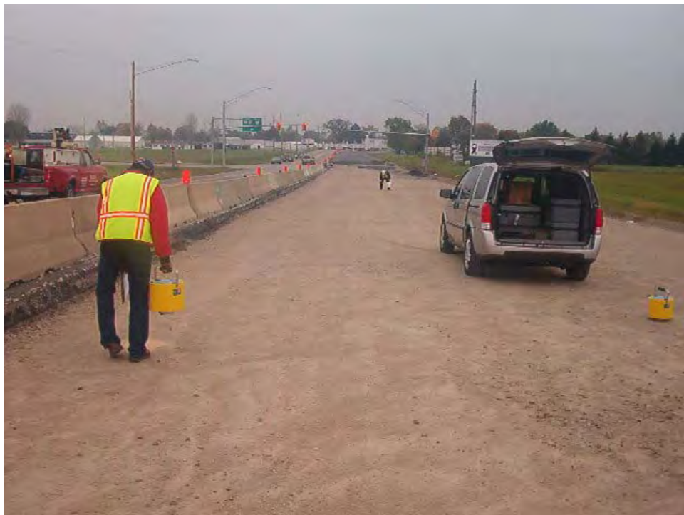
Figure B.82. NDT Testing of the Crushed Stone Base with Multiple GeoGauges and the DSPA Along SR-53 in Ohio
