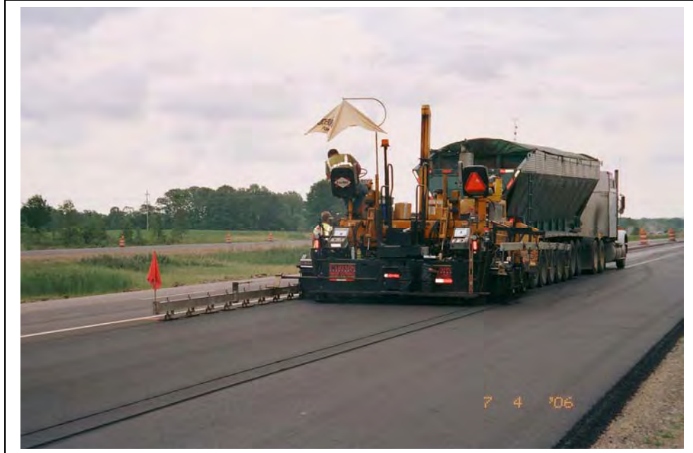
Figure B.37. General View of the Paving Operation Along I-75 of the Traffic Lane and Shoulder Near Saginaw, Michigan
