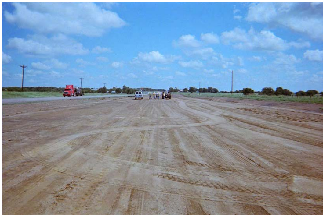
Figure B.25. Overview of the Area and Condition of the Subgrade that was Tested along the Texas SH-21 Widening Project, East of Caldwell, Texas
