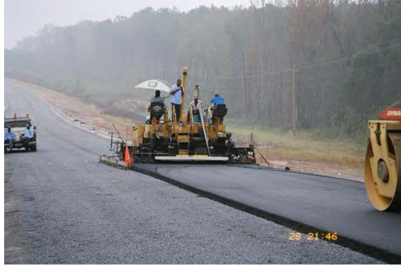
Figure B.11. Placing the HMA Base Mixture Within Section 3 on Top of the Permeable Asphalt Base Layer Along US-280; North of Opelika, Alabama (refer to Figure B.12)
