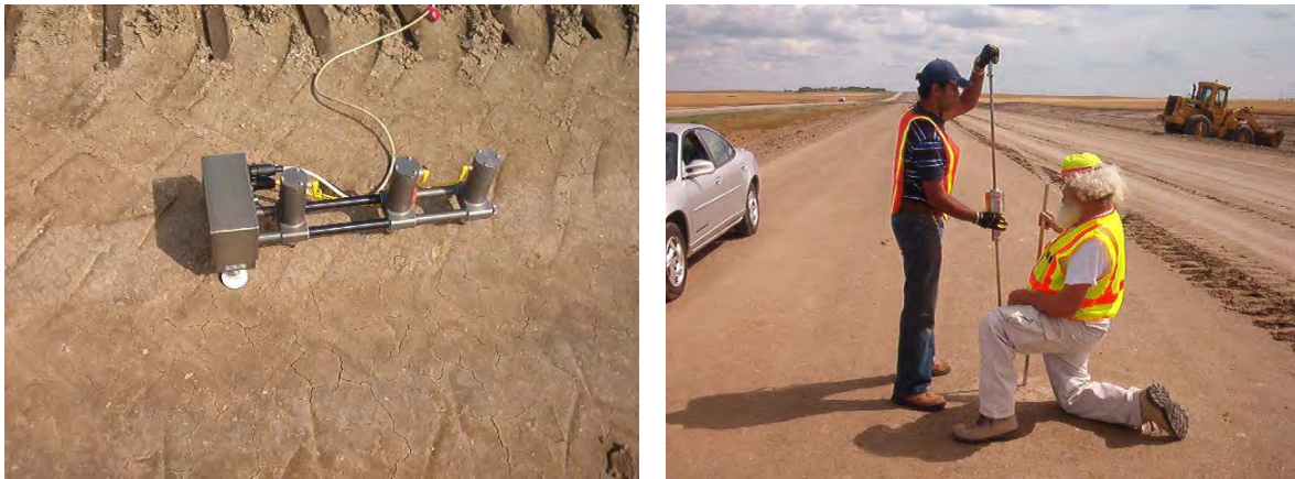
Figure B.42. Condition of Subgrade Layer Tested Along Route 2 Near Ray, North Dakota
