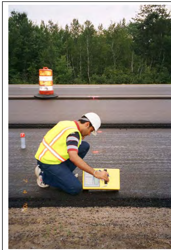
Figure B.38. PaveTracker Non-Nuclear Density Gauge Being Used Along the Shoulder of the I-75 Rehabilitation Project, Near Saginaw, Michigan
