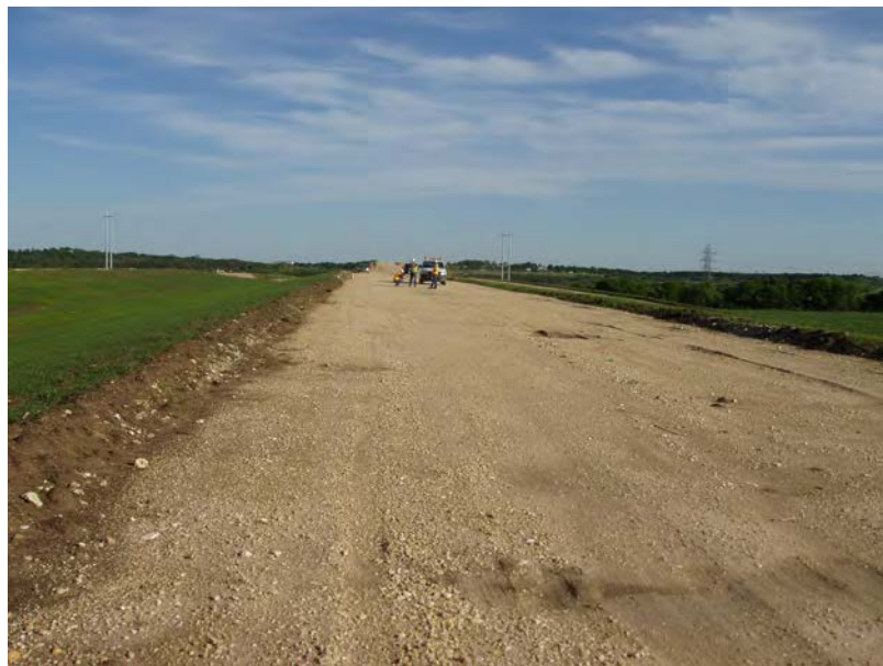
Figure B.21. Surface Condition of the Thick Improved Granular Embankment Tested Along SH-130, Near Georgetown, Texas
