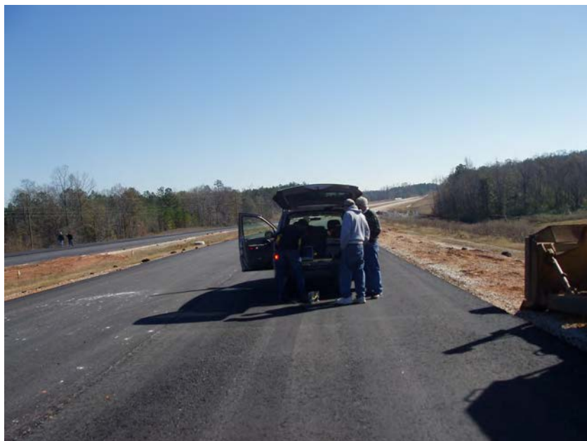
Figure B.15. Eastbound Lanes of US-280 HMA Base Mixture Testing (refer to Figure B.14)
