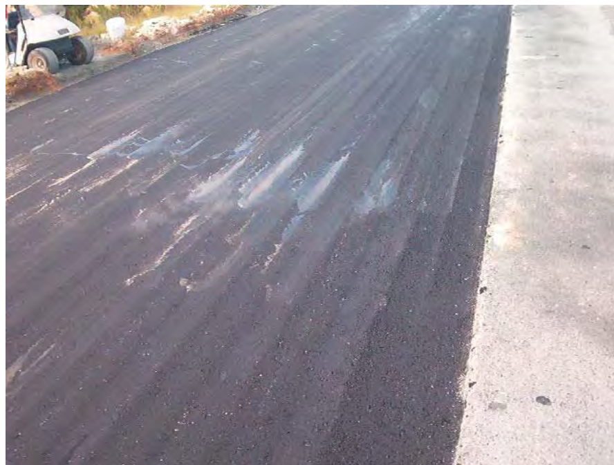
Figure B.78. HMA Compacted Using a Pneumatic Roller in the South Carolina Section S-11 at NCAT
