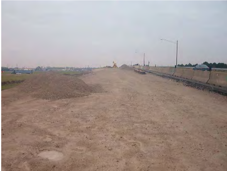
Figure B.81. Crushed Stone Base Section Tested Along US-53 at Fremont, Ohio
