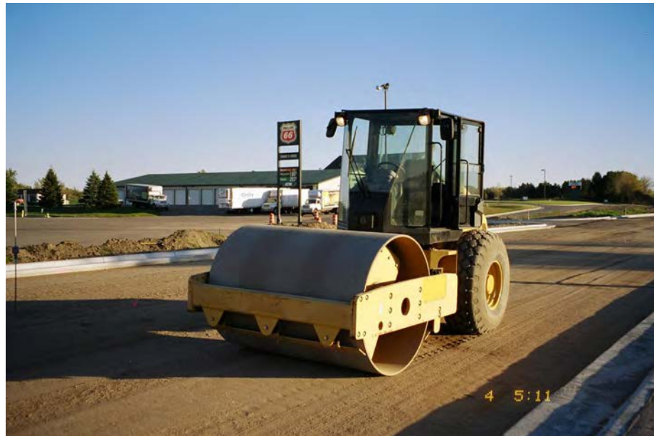
Figure B.5. Caterpillar IC Roller Used to Test the Stiffness and Uniformity of the Class 6 Base Material Along the TH-23 Project Near Spicer, Minnesota (refer to Figure B.3b)
