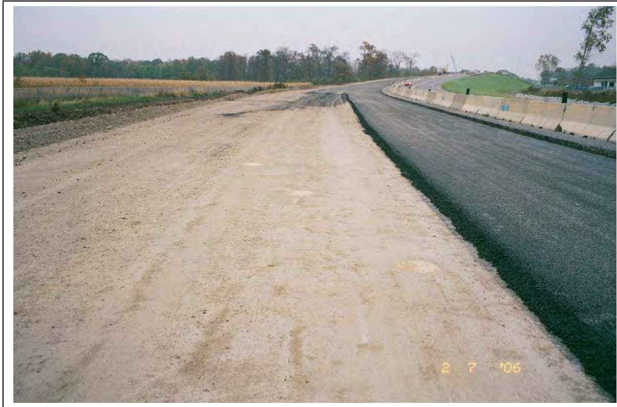
Figure B.79. New Construction Project Along SR-53 Near Toledo, Ohio Included in the Part B Field Evaluation
