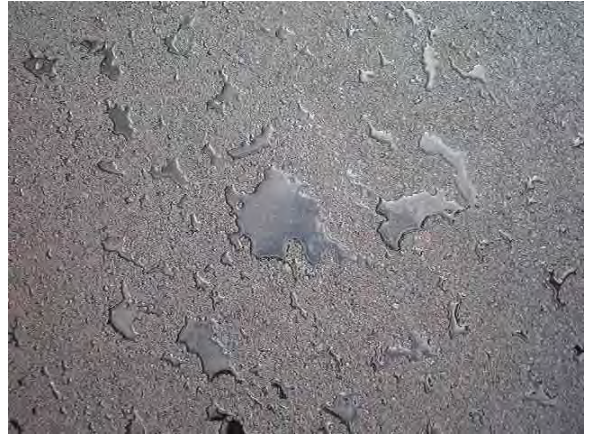
b) Close-up view of Section 1 after rain
