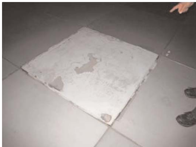
Figure 3-2. LGA arrestor: peeling paint.
