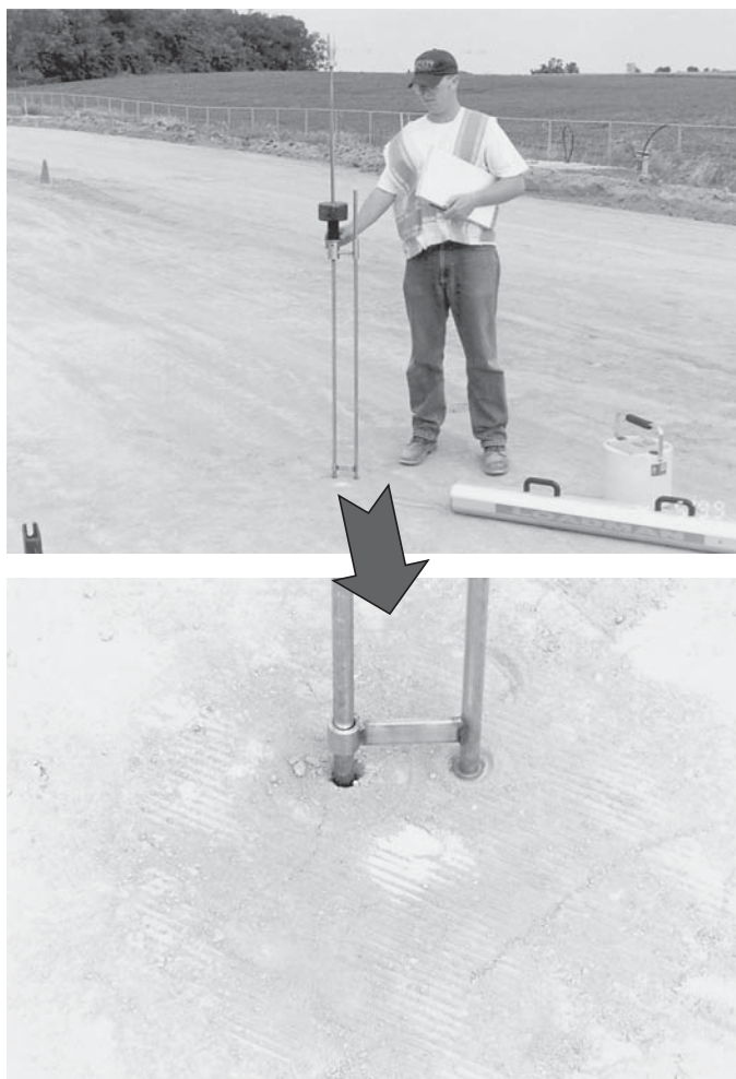
Figure 8. Manual DCP in operation (courtesy of Minnesota Road Research Section, Office of Materials, Minnesota DOT).
