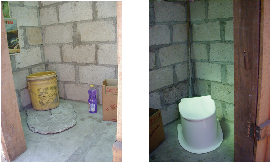
FIGURE 7-1 Examples of pit latrines and composting desiccating toilets from various water interventions. Left figure: Side of double vault composting latrine in Guatemala not in use, sealed with concrete cap. Right figure: Side of double vault composting in Guatemala in use, with toilet seat installed.
