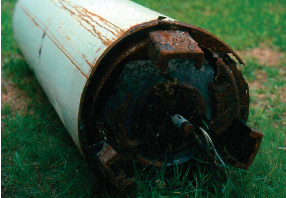
FIGURE 1-8 Corroded residential hot water heater. Courtesy of Richard Griffin.
