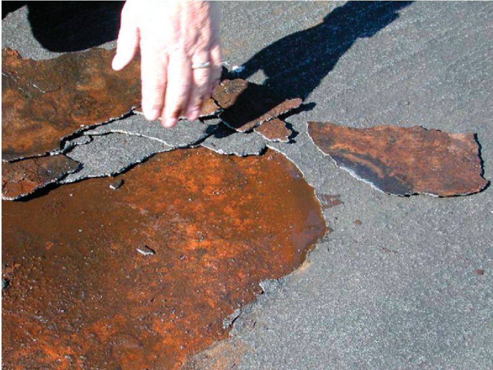
FIGURE 1-10 Corrosion on the flight deck of a naval aircraft carrier.
