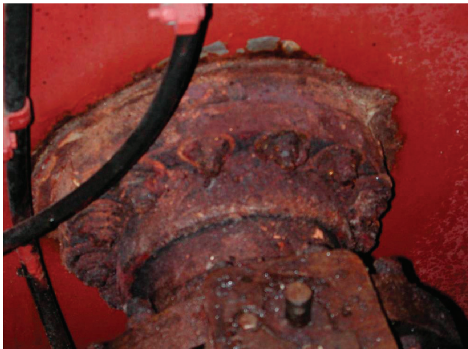
FIGURE 1-2 Corrosion under insulation in the bilge area of a naval ship.
