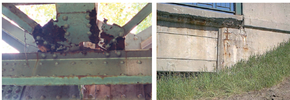
FIGURE 1-6 Examples of corrosion on various bridges. Left : corrosion on the historic Devil's Elbow Bridge on Missouri Route 66. Courtesy of Conor Watkins, Missouri University of Science and Technology. Available at http://www.rollanet.org/~conorw/cwome/article51&52combined.htm . Right : Rebar corrosion, bridge on 401 Highway in Ontario, Canada. Courtesy of Tim Mullin. Available at www.corrosion-club.com/rebarimages.htm .
