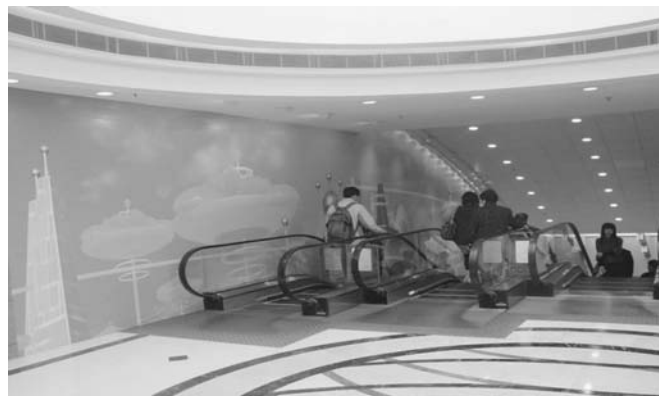
Figure 1 High Speed Escalators at MTR Station.
