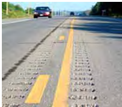
Exhibit 2-11 Centerline Rumble strips (Photo: MnDOT)
