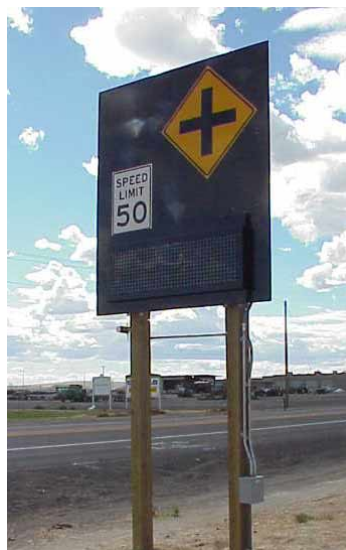
Exhibit 3-15 Dynamic warning sign installed by WSDOT.
