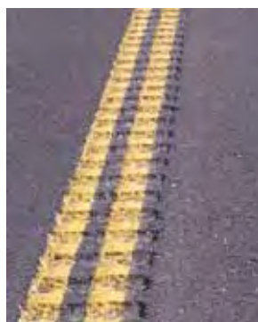
Exhibit 2-13 Centerline Rumble Strips Extending into the Travel Lane (Photo: Torbic et al.)
