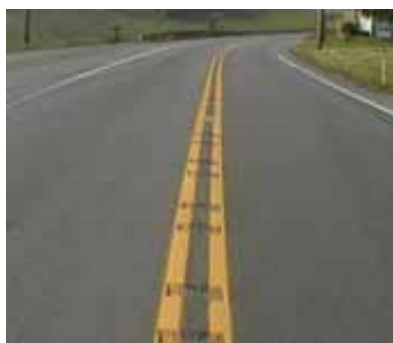
Exhibit 2-12 Centerline Rumble Strips on the Centerline Pavement Markings (Photo: Torbic et al.)
