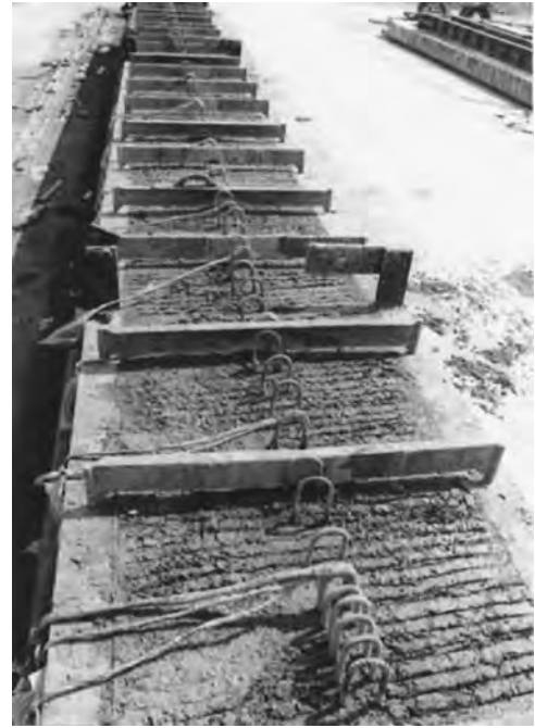
Figure 45. Roughening of surface of top flanges.
