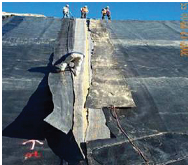
FIGURE 4.2 GCL seam separation at a California landfill. SOURCE: County of Riverside (2004).
