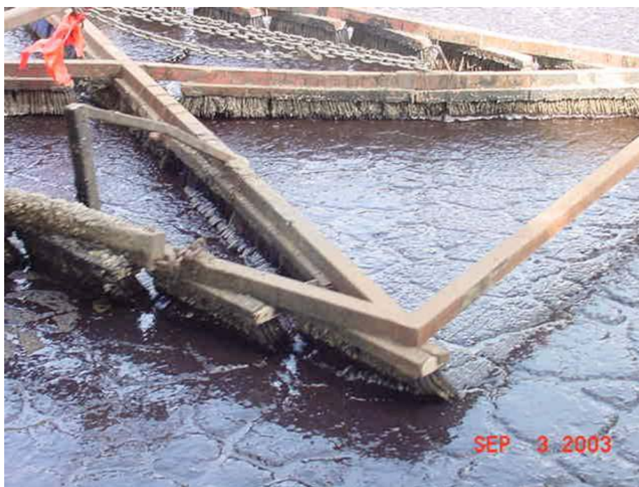
FIGURE 7 Fatigue cracks sealed with scrub broom before chipping.
