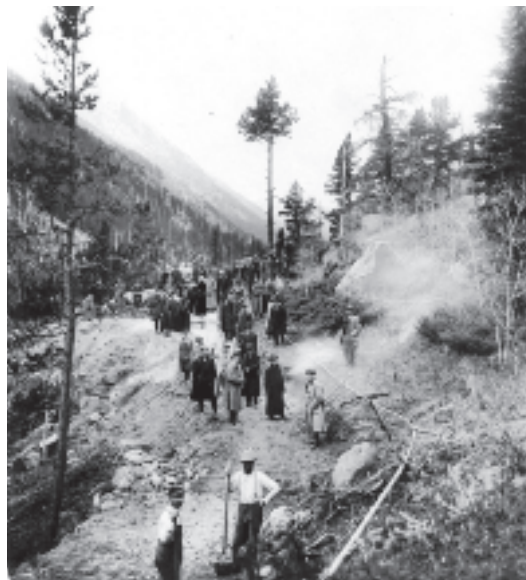
Construction of Fall River Road, the first road to cross the Rocky Mountains in northern Colorado, September 1915.
