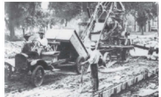
Road construction in Michigan, one of the first states with an engineer highway commissioner.
