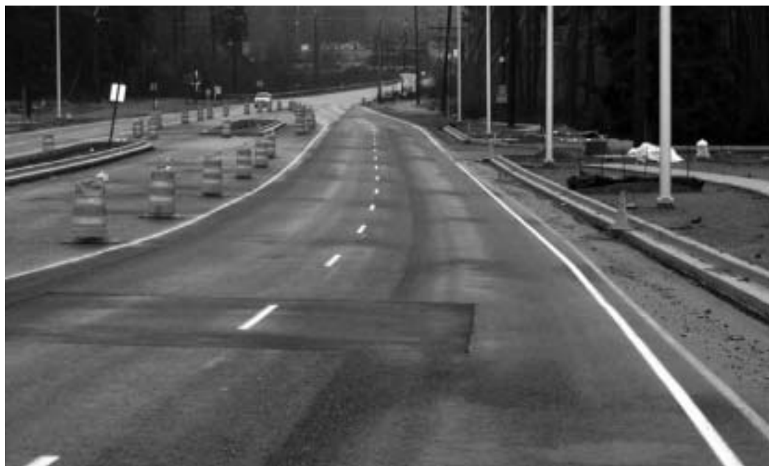
FIGURE 1 Cyclic low-density spots just after construction.
