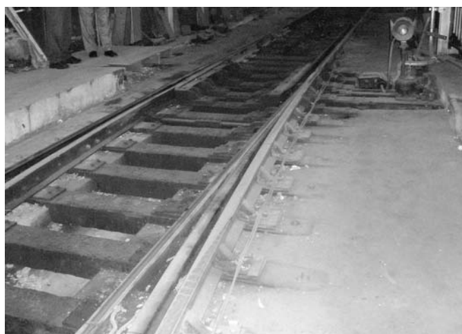
Figure 2-15. Fully guarded switch in Penn Station.
