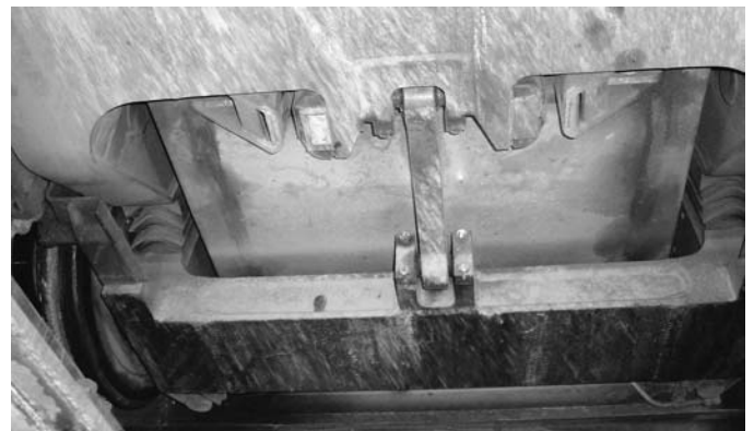
Figure 2-12. Lateral bump stops on the center truck (NJ TRANSIT Kinki Sharyo LFLRV).
