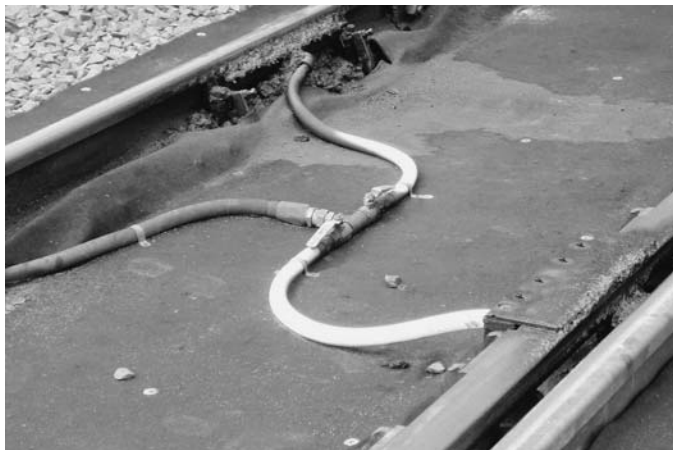
Figure 2-17. Friction conditioners for rail flange and guide rail in the workshop area.
