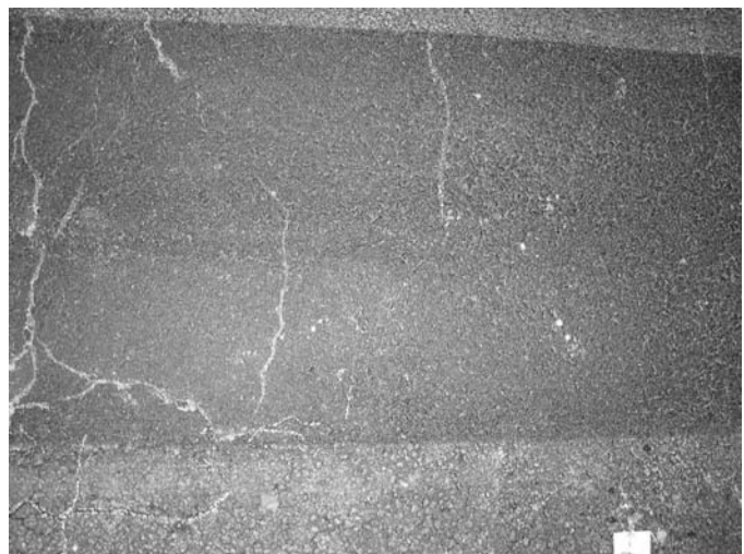
Figure 13. CA-2 test section after 80,000 wheel passes.
