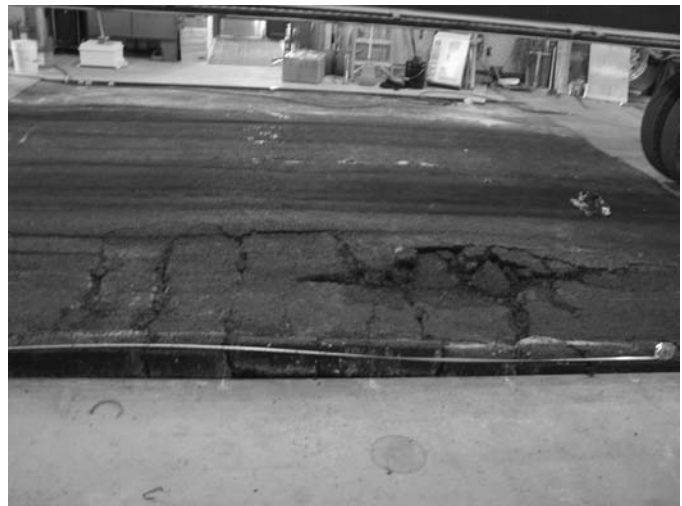
Figure 12. CA-3 test section after 1,000 wheel passes.
