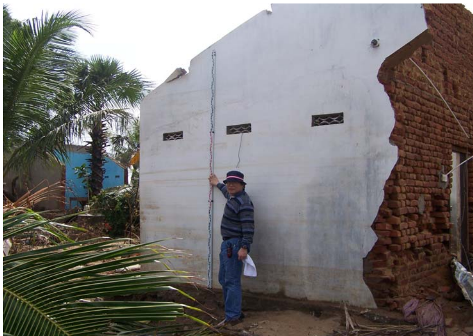
Figure 1. Mud lines on a destroyed Sumatran building. Photograph by Patrick Lynett, Texas A&M University
