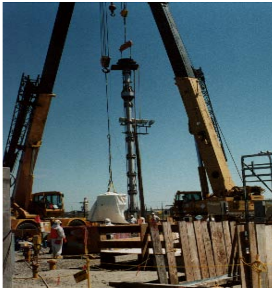
FIGURE III-2 Mixer pump used in Hanford Tank AZ-101. SOURCE: Gasper, 2003.
