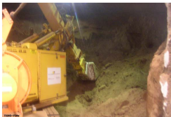
FIGURE G-16 Pneumatic (vacuum) retrieval from the top of Silo 3 at the Fernald facility in Ohio ( left ) and mechanical retrieval tool (the Excavator) operating from an opening in the wall of the silo ( right ). The wall of the Silo is visible at the right border of the frame. SOURCES: Left: www.nukeworker.com; right: Beckman, 2006.
