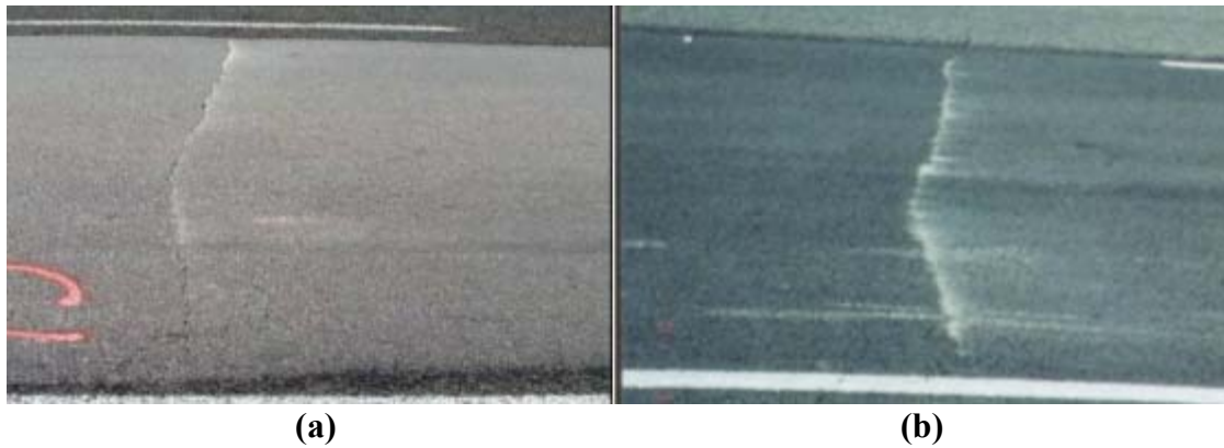
FIGURE 7 Crack developments on remixer section (US-84): (a) before remixer process (US-84) and (b) 2 months after remixer process (US-84).
