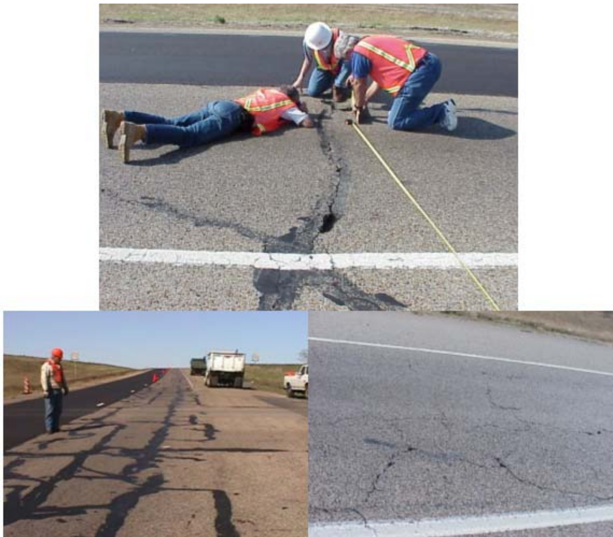
FIGURE 5 Pavement conditions before overlay on the HIP section (US-175).
