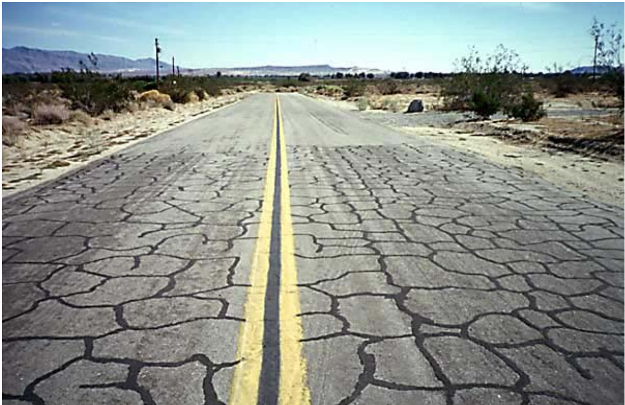
FIGURE 1 Crack sealing normally required on desert roads.
