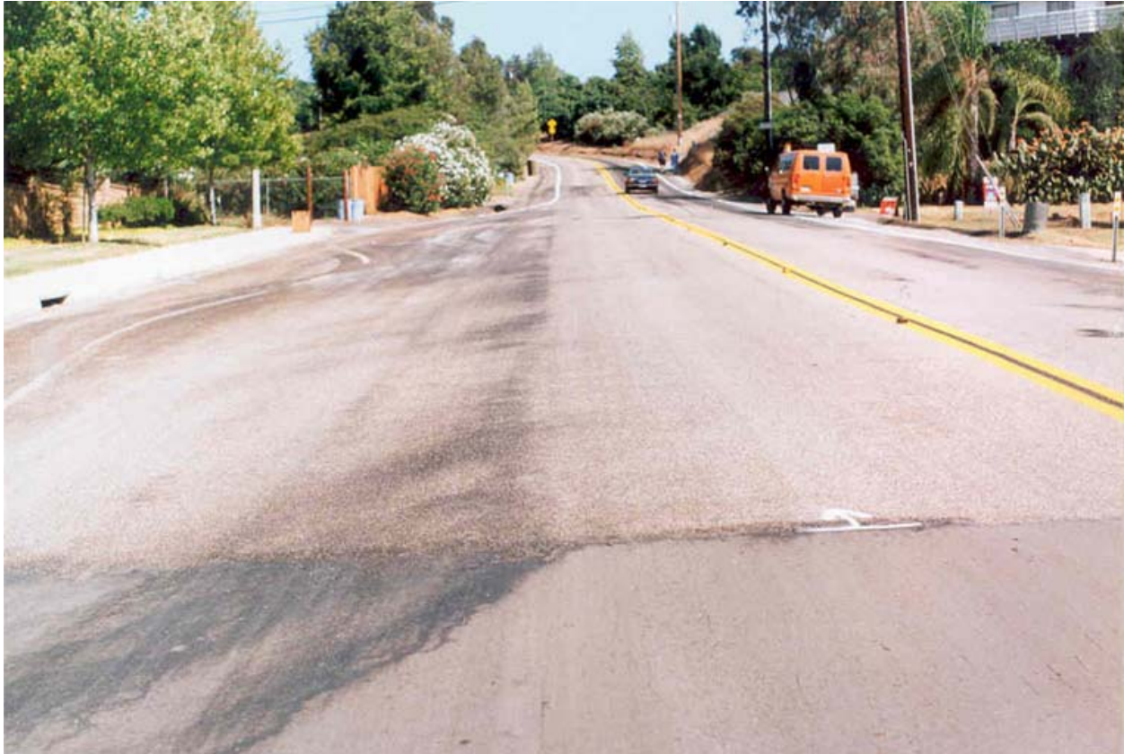
FIGURE 4 Effects of a rain storm that occurred within 24 h after chip sealing.
