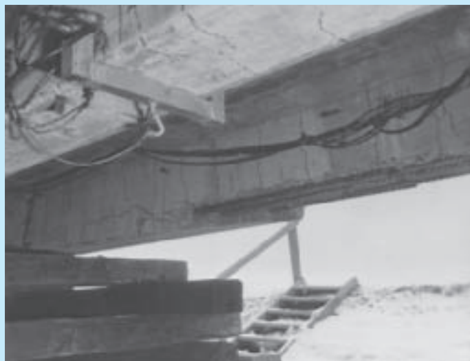
Fatigue failure of reinforcing bars in a reinforced concrete bridge.
