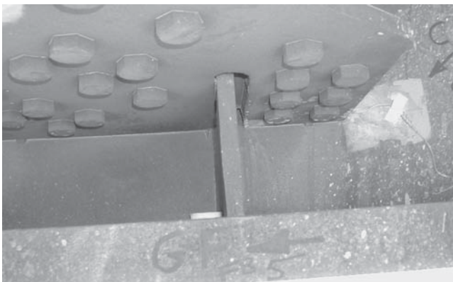
FIGURE A3 Fractured girder of the Hoan Bridge in Milwaukee (top) and view of critical shelf plate detail featuring intersecting welds.
