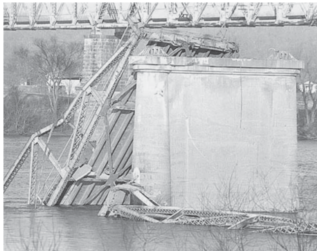
FIGURE 1 Collapse of Point Pleasant Bridge.
