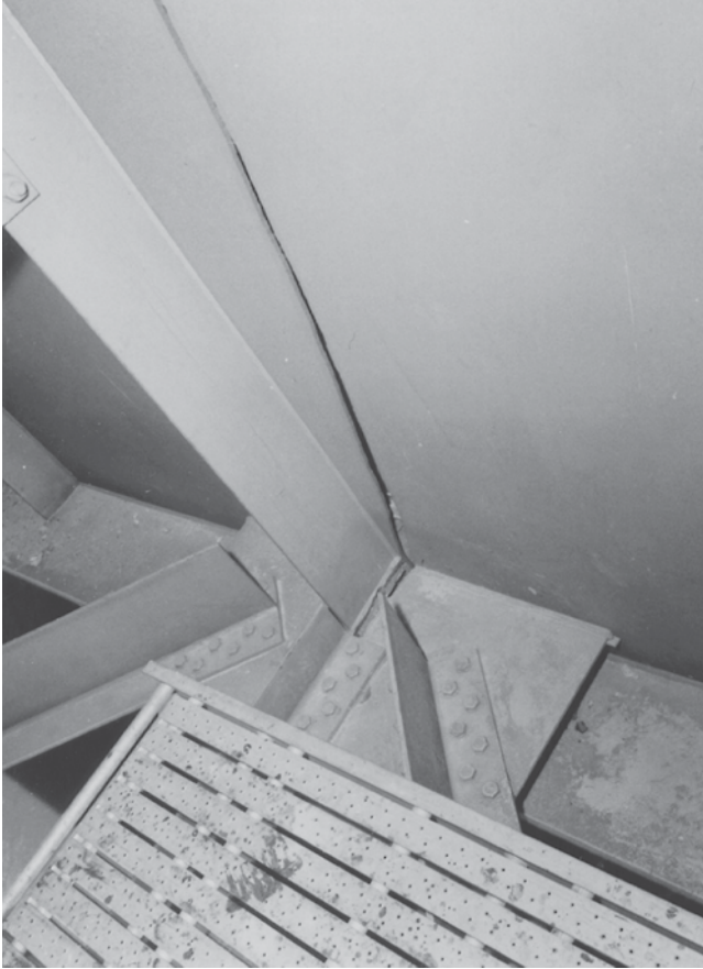
FIGURE 16 View of cracked girder in two-girder span of Lafayette Street Bridge in St. Paul, Minnesota, as an example of a bridge that is sufficiently redundant to avoid collapse despite a fracture of the tension flange and the web of one girder.
