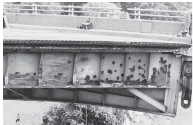
FIGURE 4 Collapse of Mianus River Bridge. (Courtesy: John W. Fisher.)
