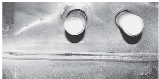
FIGURE A5 Example of indication from dye penetrant inspection.
