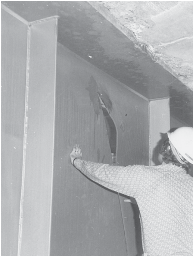
FIGURE A12 Full-girder-depth fatigue crack of Lafayette Street Bridge in St. Paul, Minnesota.
