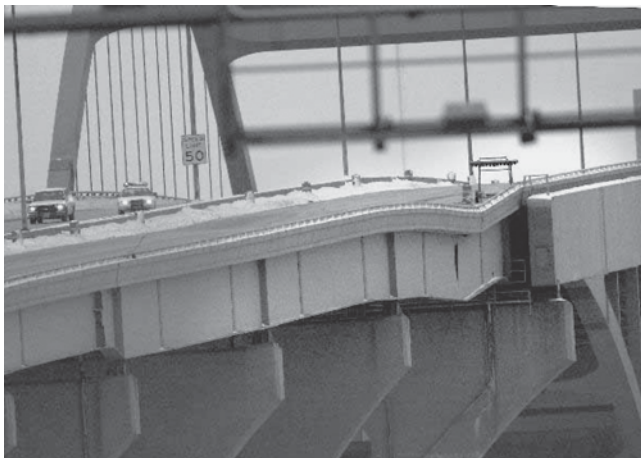
FIGURE 9 Example of bridge deck acting as catenary with hinge at fracture location in end span of the approach spans of the Hoan Bridge in Wisconsin—two of the three girders had full-depth fractures in December 2000.
