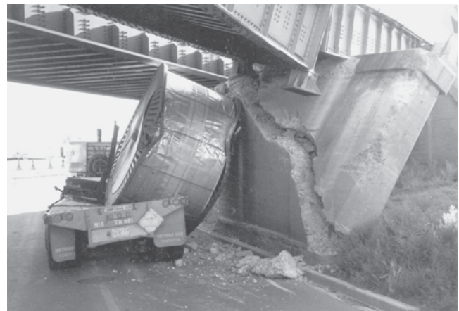
FIGURE 7 Example of vehicle–bridge collision causing collapse owing to nonredundant substructure. (Courtesy: Robert Sweeney.)
