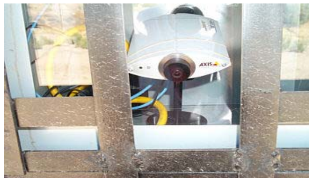
FIGURE 2-5 Gaging station on the flashflood-prone Santa Cruz River in Arizona includes a webcam to transmit hourly photos to warn of floods in the otherwise dry channel. SOURCE: USGS ( http://az.water.usgs.gov/webcam/9482500_cam/cam_09482500.html ).
