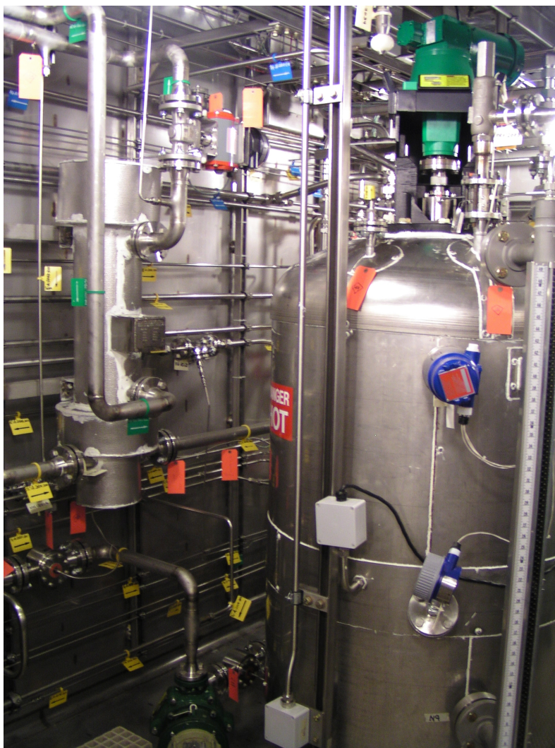
FIGURE 2-4 Reactor vessel in the chemical process trailer. In this view note the proximity of the reactor vessel to the wall of the trailer and the consequent restricted access for inspection, maintenance, or repair of the pumps and instrumentation.
