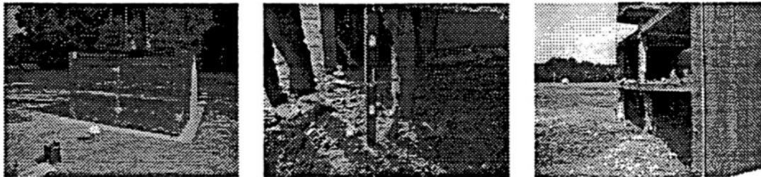
Figure 4: In-Fill Walls, Severe Damage to Column
