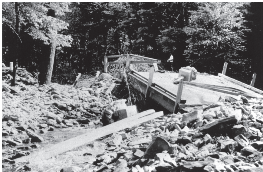
Flood damage to bridge and road. Note person on bridge for scale. Photo courtesy of U.S. Geological Survey.
