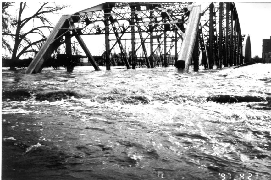
Flood overtopping Sorlie Bridge, Grand Forks, ND, during spring of 1997. Photo courtesy of U.S. Geological Survey.
