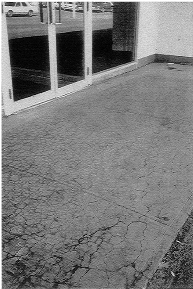
FIGURE 1–14 Cracking in concrete paving caused by an expansive reaction between the aggregate and the alkalis in the cement paste. Source: Hansson, 1995.
