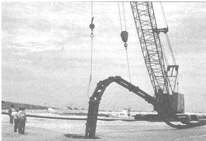
FIGURE F-1 Sand bypassing at Indian River Inlet, Delaware. Jet pump positioned by crane (from Wayne Young, Marine Board, National Research Council).
