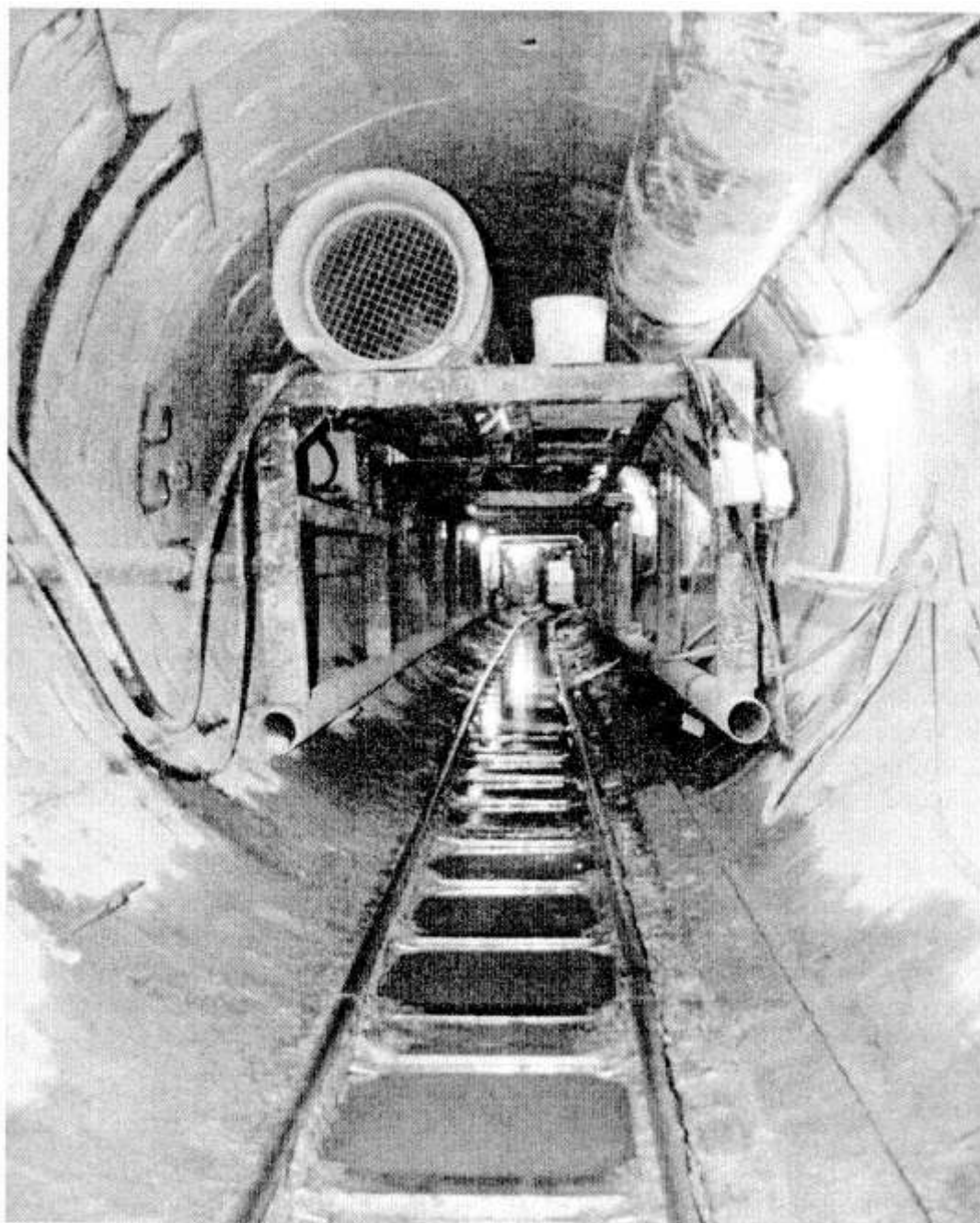
Figure 3 Tunnel ventilation system using fully reversible, explosion-proof fans.
