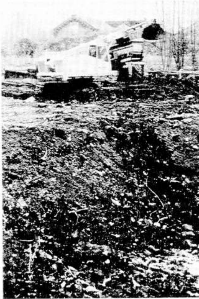
Excavation of a contaminant source area at a former coal gas plant. Courtesy of the Johns Hopkins University, Department of Geography and Environmental Engineering.
