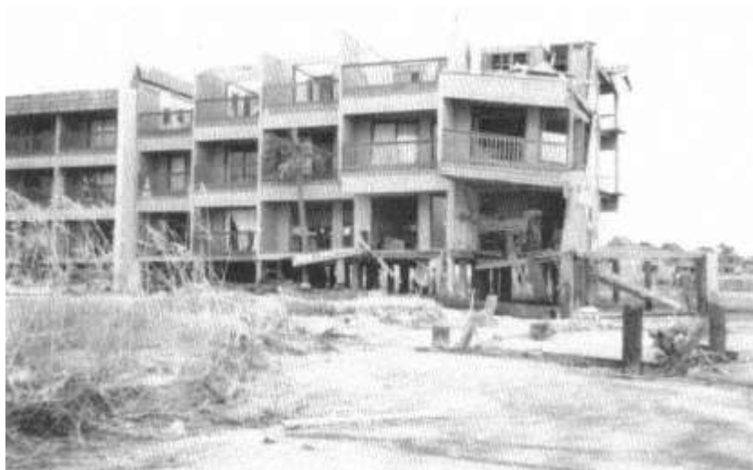
Figure 12-14a Modular unit construction with poor connections.
