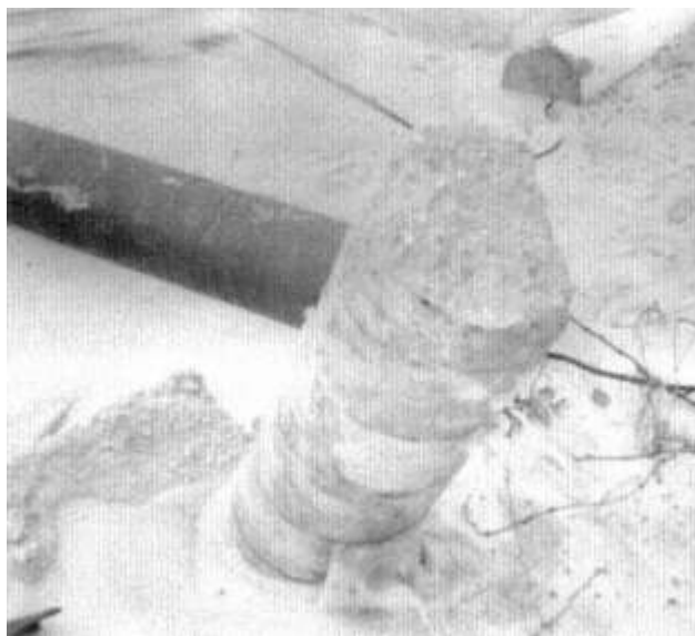
Figure 12-11b Broken piers revealed inadequate placement of reinforcing bars.
