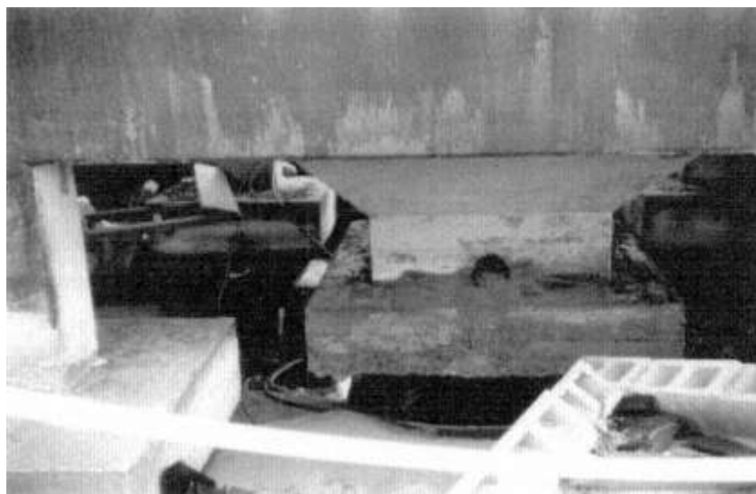
Figure 12-9 Bulky shallow footing promoted scouring around it.
