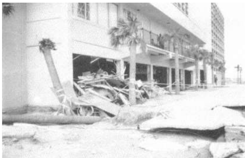
Figure 12-2 Water damage to the ground-level units and waterfront amenity facilities at the Holiday Inn on Folly Island. This damage was typical of that suffered by highrise hotels and condominiums.
