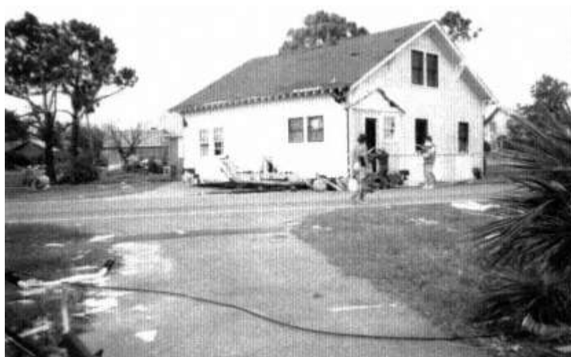
Figure 12-7a Structure built on slab floated away from foundation and deposited 100 ft away.
