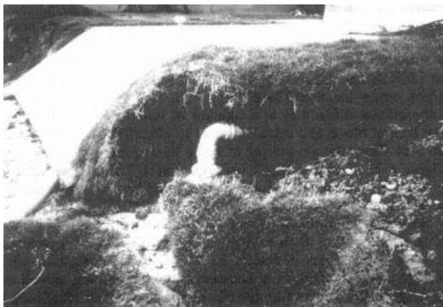
Figure 5-14 Wastewater pipes, Isla Verde.
