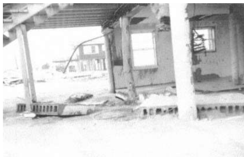
Figure 12-11a Poured concrete piers buckled under lateral load.
