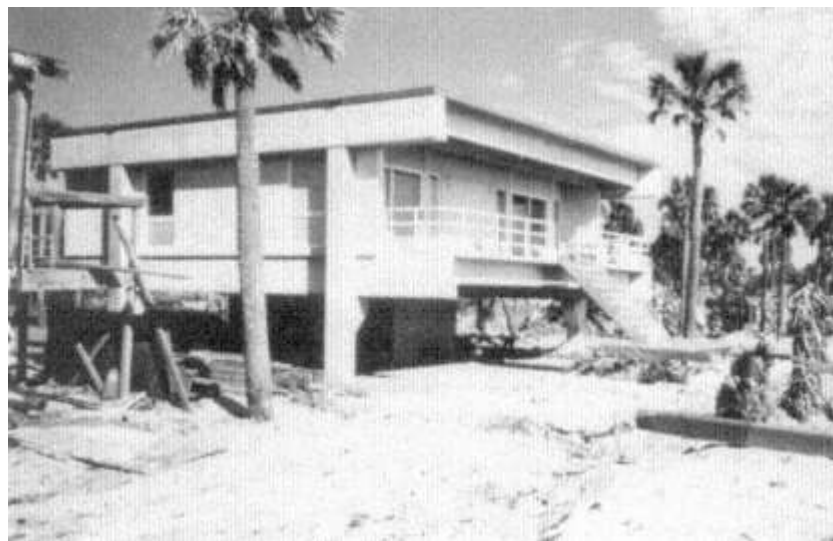
Figure 12-1 A concrete residential structure on Folly Island survived with in an area of heavy destruction.
