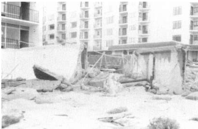
Figure 12-16 Overtopping induced seawall failure.
