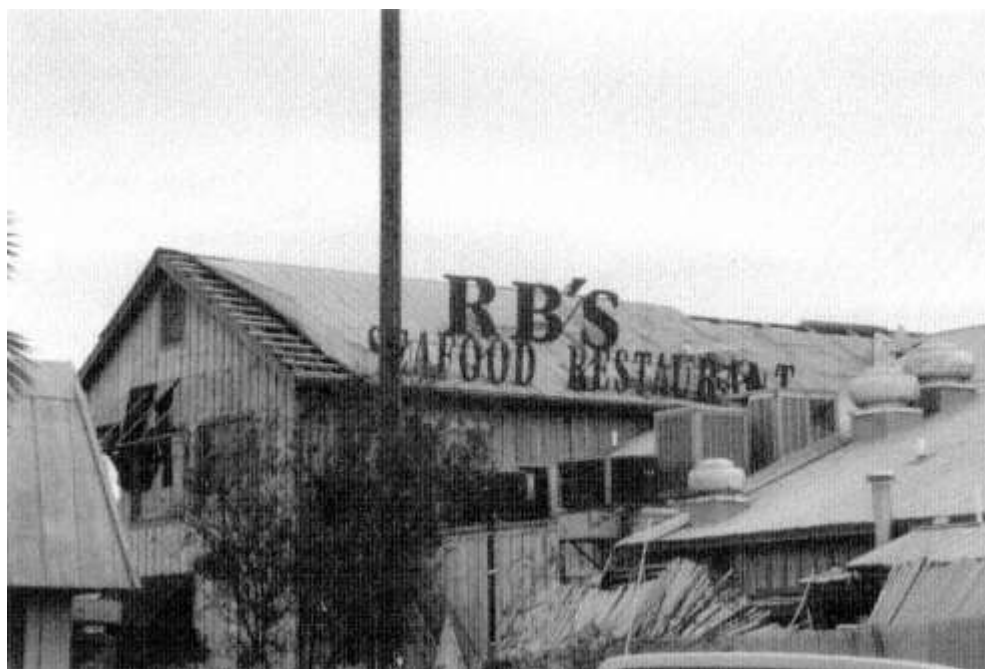
Figure 13-3 Typical damage to metal roof coverings.
