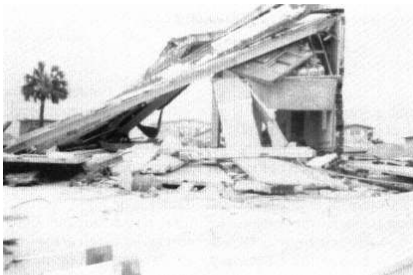
Figure 12-5 A two-story concrete residential structure collapsed under its own weight because of weak foundation (Garden City).
