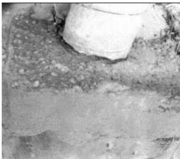
Figure 12-12 Bad joint between pier and footing was a common cause of failure.
