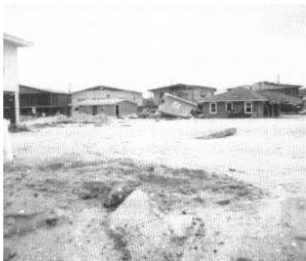
Figure 12-4 Sand overwash on second row of houses (north of Waccamaw Avenue), Garden City.
