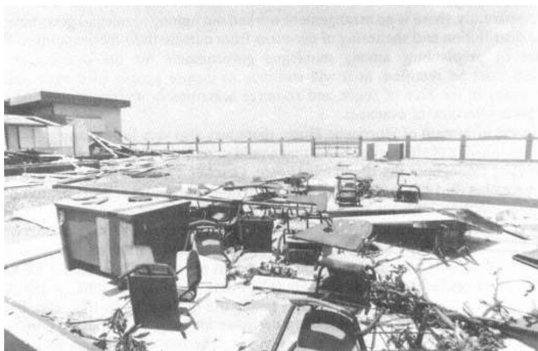
Figure 3-2a One view of the Rosendo Matienzo Cintron School in Luquillo, Puerto Rico, used as a shelter during Hurricane Hugo (first photo).
