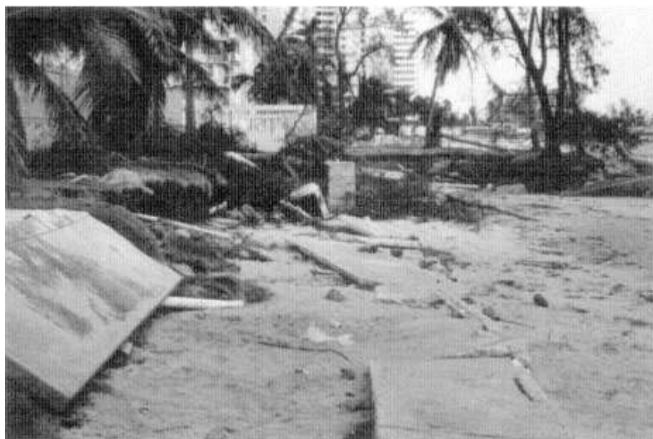
Figure 6-15 Punta el Medio area in Isla Verde showing unearthed water and waste pipes.
