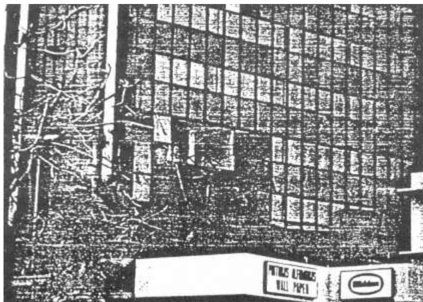
Figure 4-32 Damage to curtain wall near street level, San Juan.
