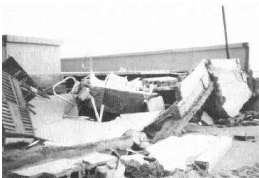
Figure 12-17 Underdesigned return wall was common.
