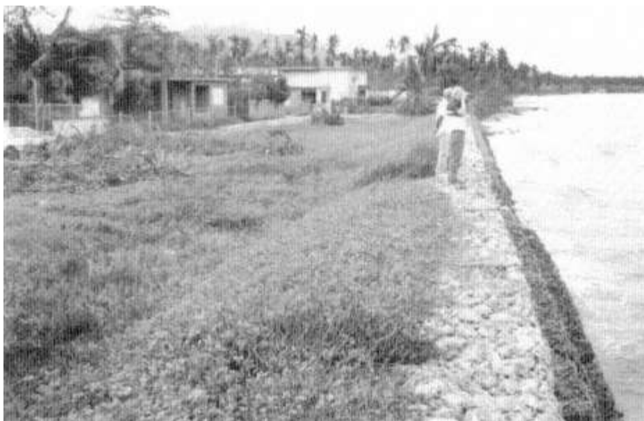
Figure 6-19 The gabion wall at Playa de Humacao. The beach is gone, and waves will now begin to attack the wall directly. Some beach rebuilding is expected naturally, though how much is impossible to predict.
