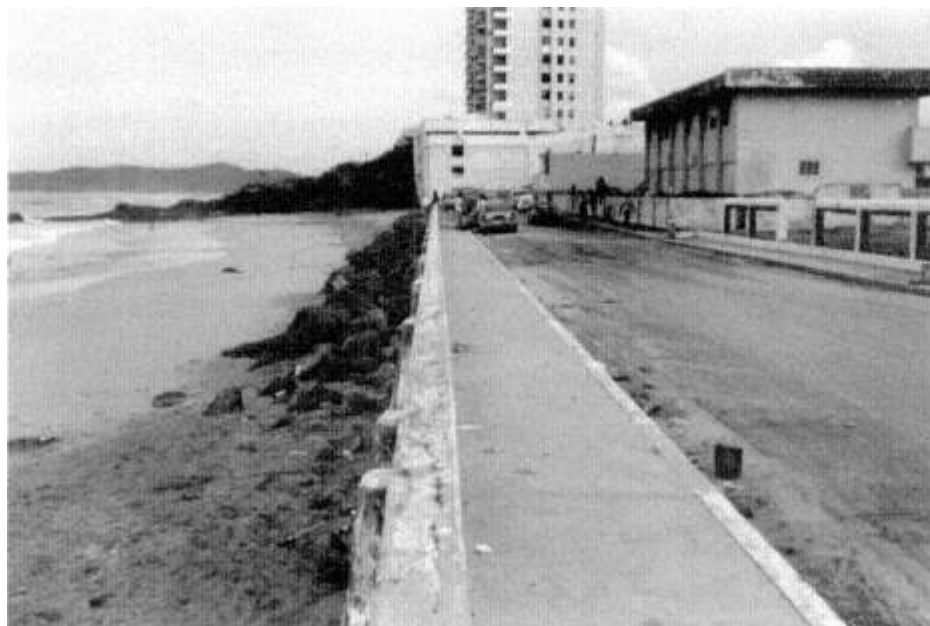
Figure 6-3 Luquillo shorefront showing seawall that had reportedly fallen during Hugo. Storm surge and wave heights near the time of passage of the eye were determined by observing water levels on the distinctive rock formations.
