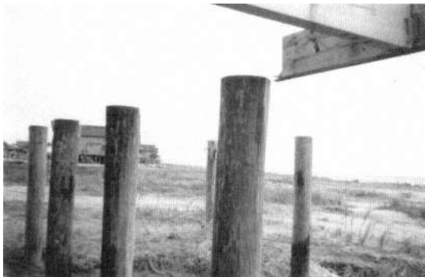
Figure 12-14b The end unit of the modular structure simply disconnected from the piles.
