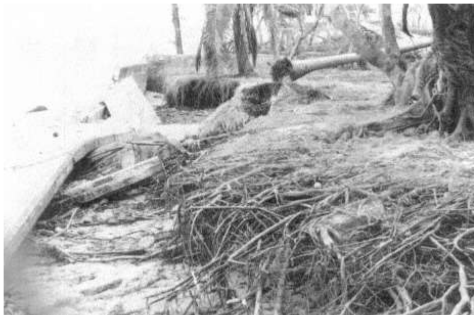
Figure 6-13 Shorefront in Punta las Marias, Calle Almendro, showing unearthed tree roots, toppled seawall, and shoreline retreat.
