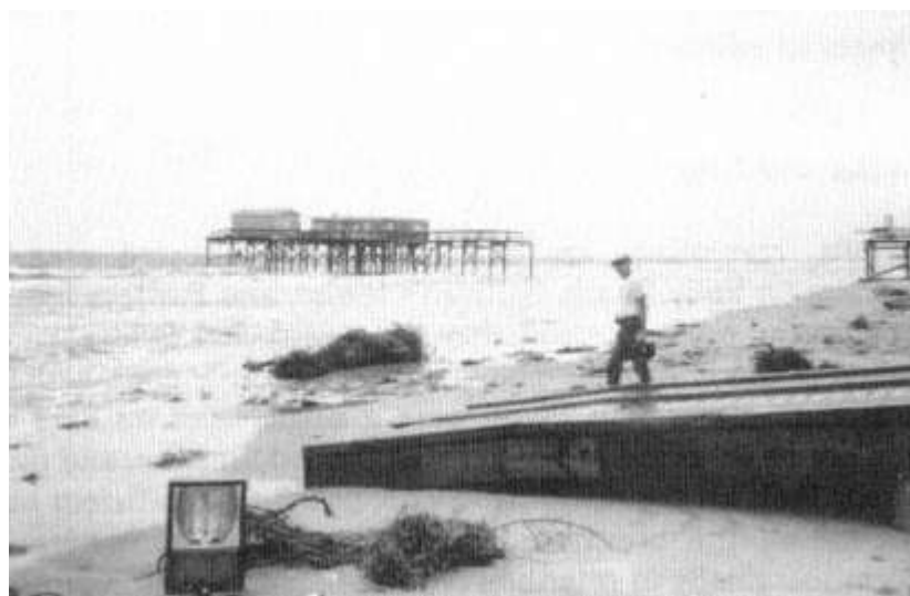
Figure 12-18 Piers with midsection missing revealed the location of maximum dynamic force to be in surf zone.
