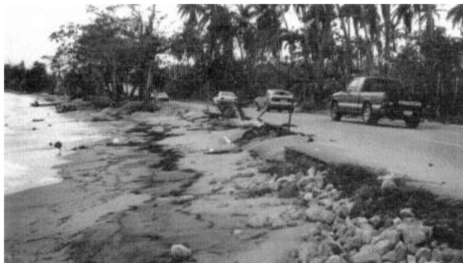
Figure 5-11 Undercutting of pavement by wave action on Route 3, north of Humacao, Puerto Rico.
