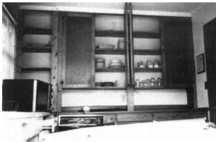
Figure 12-7b The arrangement inside the kitchen of the same structure remained undisturbed.
