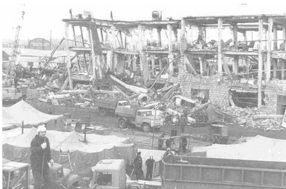
FIGURE 5.9 Earthquake damage to a precasting plant in Axtoran (near Leninakan), Ukraine. This plant made building components for the precast, reinforced-concrete buildings in Leiniakan. Note the collapsed precast-prestressed concrete trusses. Photograph by Fred Krimgold; reproduced from Earthquakes and Volcanoes 21(2) , p. 73.
