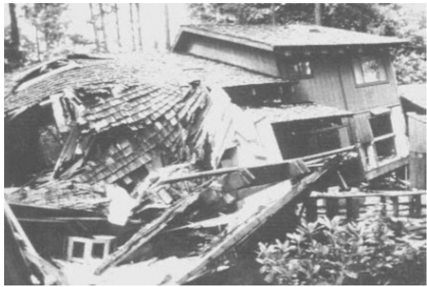
FIGURE 1-17 Collapsed house at Boulder Creek.
