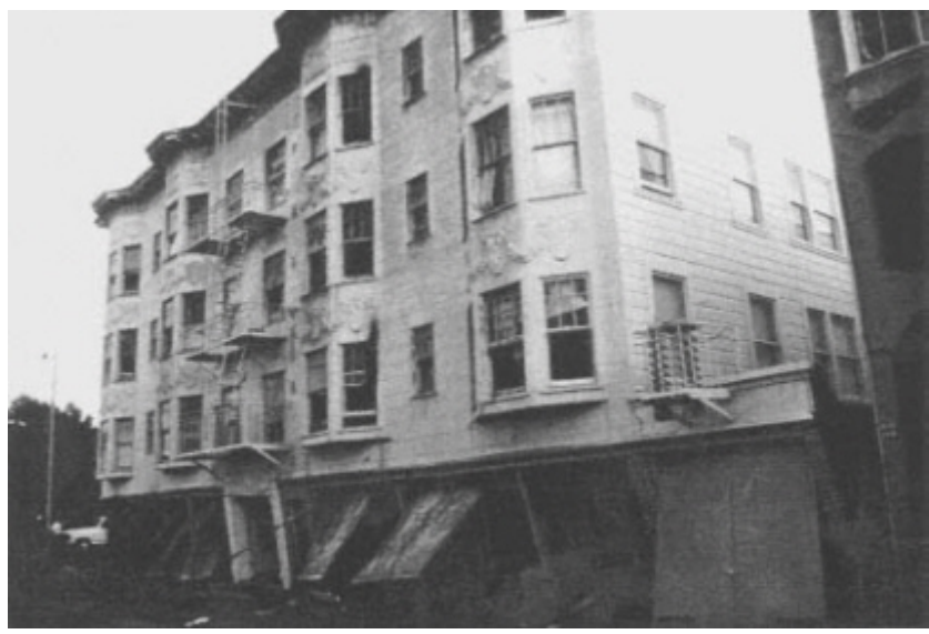
FIGURE 1-12 Multistory building in the Marina District.
