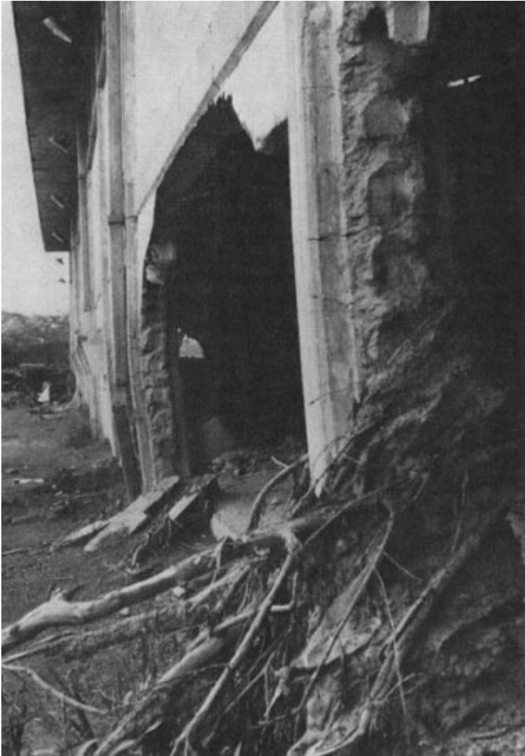
Figure 3.2 Reinforced pillars on downstream wall of the building in Figure 2.15 . The concrete block fill-in has been nearly entirely removed. Pillars are cracked and bent in the downstream direction. (Photo by R. Updike, USGS.)
