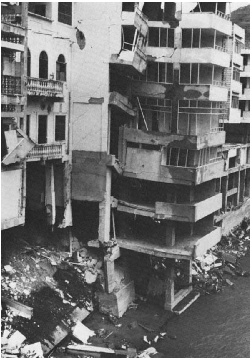
Figure 3.3 Foundation damage to apartment buildings in Honda along the channel of the Gualí River. (Photo by R. Updike, USGS.)
