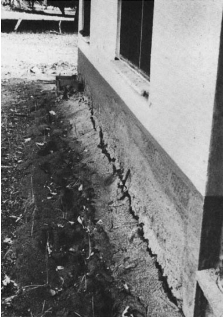
Figure 2.18 The administration building at a serpentarium 5.5 km north (downstream) from Armero. Note the high mud line on the building wall. According to trapped survivors, the mud gradually lowered to the present surface in about three days. (Photo by R. Updike, USGS.)
