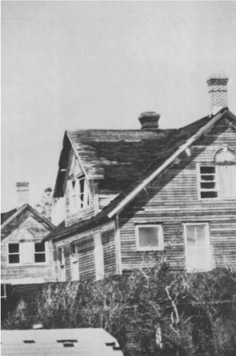
Figure 4-38 Minor damage to old military building, near Fort Gaines, Dauphin Island.
