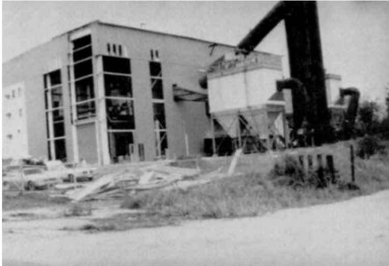
Figure C-1 Damage to cladding (side and leeward walls) of the Pascagoula Energy Recovery Facility resulting from overhead door failure.
