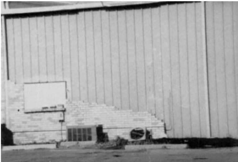
Figure C-3 Brick veneer stripped from metal building by high suction pressures.
