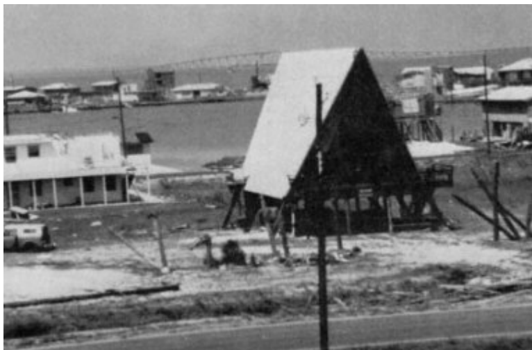
Figure 4-41 Damaged building with low-pitched roof (left) and undamaged A-frame house (right), Dauphin Island.
