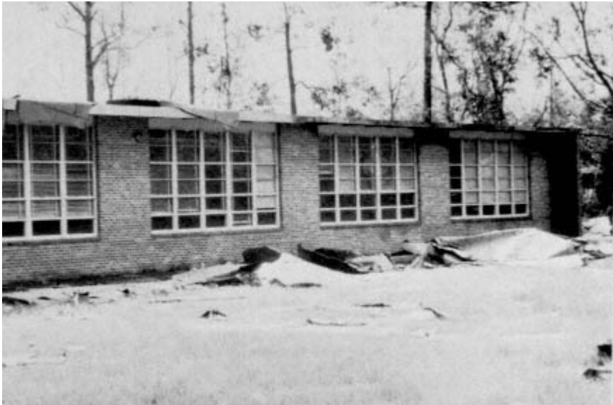
Figure 4-1 Loss of roof covering—West Elementary School.
