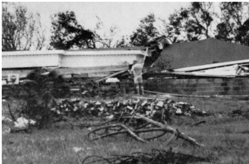
Figure 4-16 Shear failure of house, Pascagoula.
