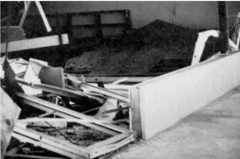
Figure 4-5 Wall-to-window-frame connection failure, Jackson Square Shopping Center, Gautier.
