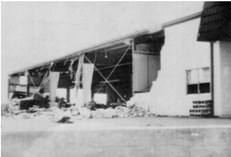
Figure C-4 Damage to unreinforced masonry wall enclosing metal building in Biloxi. Failure may have been precipitated by loss of large overhead doors. Steel framing was undamaged.
