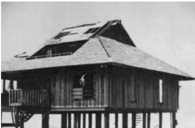
Figure 4-42 Roof damage showing the influence of roof shape, Dauphin Island.
