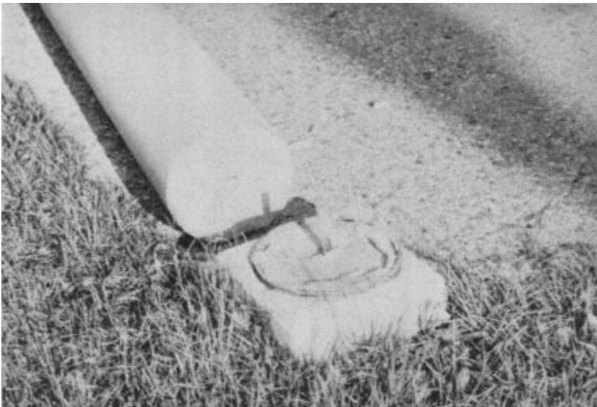
Figure 4-32 Base-to-column connection of shelter of Figure 4-31 .
