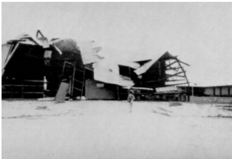
Figure C-8 End bay damage to preengineered building in Pascagoula. Note new, undamaged metal building on right.
