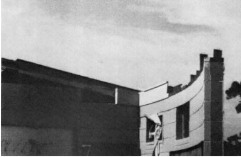
Figure 4-44 Loss of roof, Isle Dauphin Country Club, Dauphin Island.
