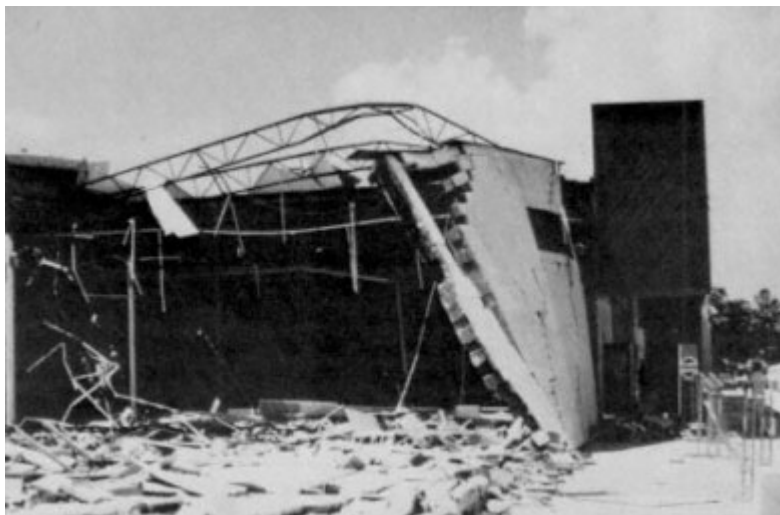
Figure 4-6 Buckling of bar joists due to roof uplift, Jackson Square Shopping Center, Gautier.
