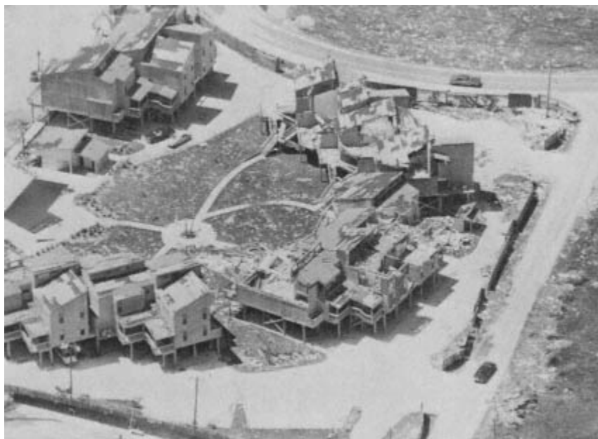
Figure 4-17 Extensive damage to Spinnaker Point Condominiums, Pascagoula. (Courtesy of The Sun/The Daily Herald , Biloxi.)
