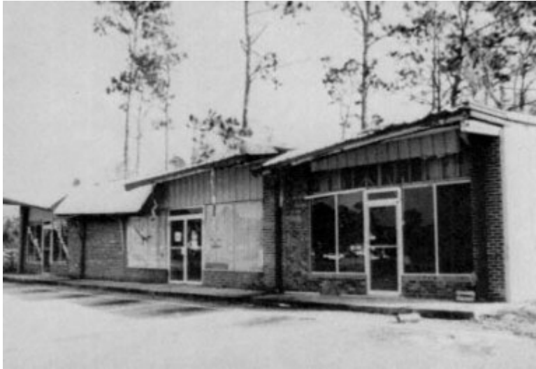
Figure C-2 Wind damage of canopy of metal building in Gautier. Note that overhang has been provided by extending roof sheeting beyond eave, a poor but common practice.
