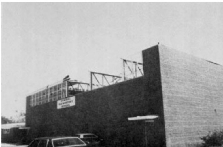
Figure A-5 Gymnasium damage, Central Elementary School, Gulfport.
