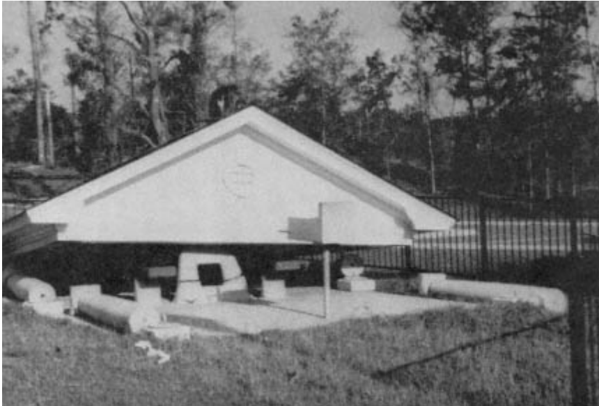
Figure 4-31 Collapsed roadside shelter at rest area on Interstate Highway 10 All units failed.
