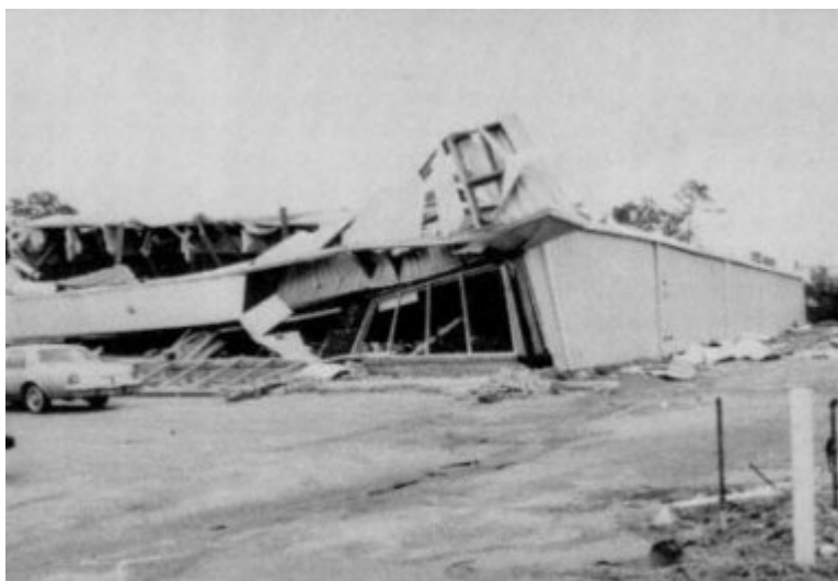
Figure C-7 Metal building system in Pascagoula. Failure due to buckling of strut purlins under combined bending and axial loading. Damage limited to first bay.
