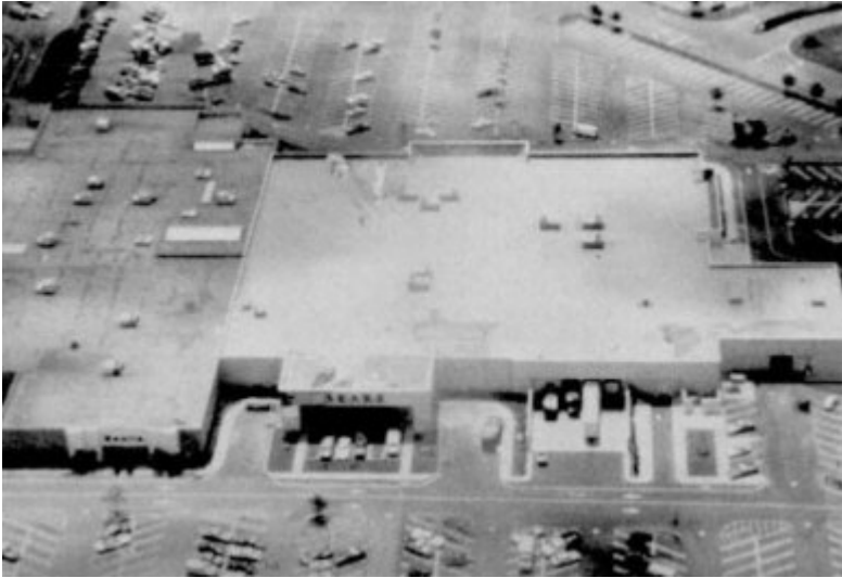
Figure 4-2 Roof membrane damage to a shopping mall, Gautier.
