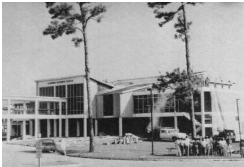
Figure 4-28 Learning Resource Center, Mississippi Gulf Coast Junior College; roof damage.
