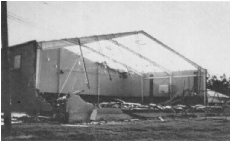
Figure A-4 Collapse of gymnasium at Dukate Elementary School, Biloxi.
