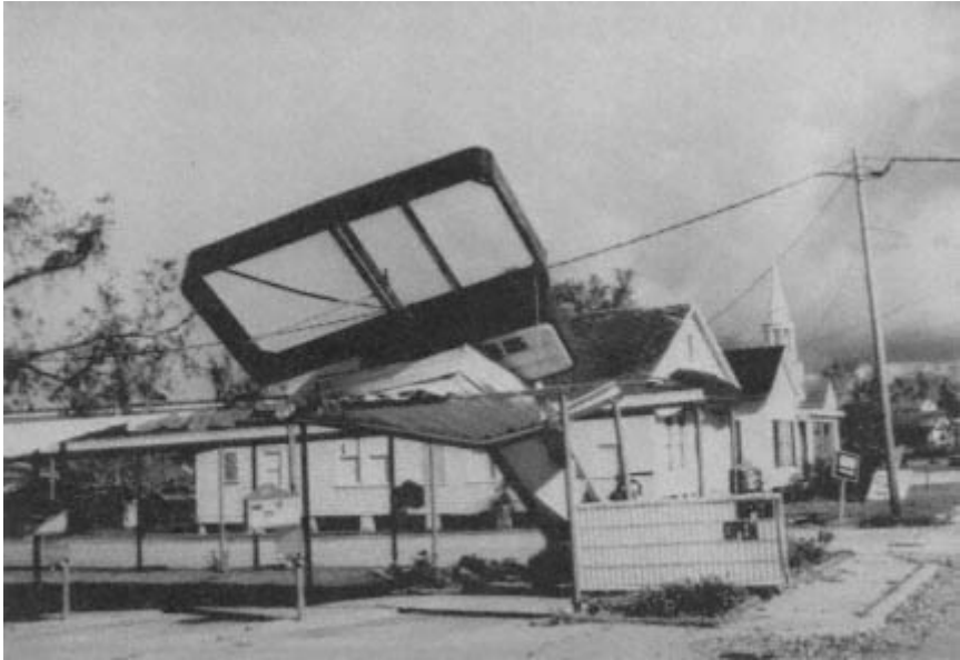
Figure 4-35 Failure of sign in Moss Point.
