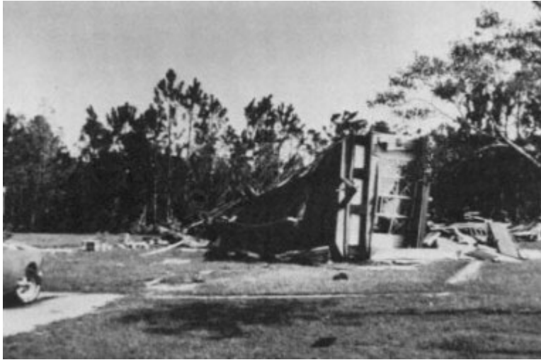
Figure 4-18 Anchor failure in mobile home, Gautier.
