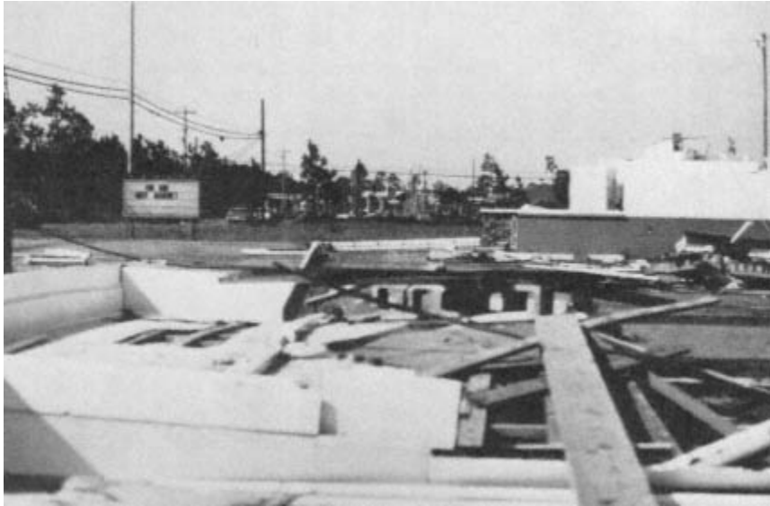
Figure 4-10 Loss of wood roof from masonry-walled building (note sign), Gautier.
