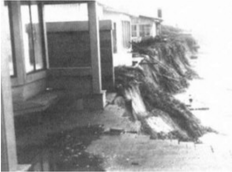
Figure 2-1 Several homes in jeopardy and vertical scarp, western end of Seadrift, Stinson Beach, California, January 27, 1983. SOURCE: Photo provided by Robert E. Wiegel.
