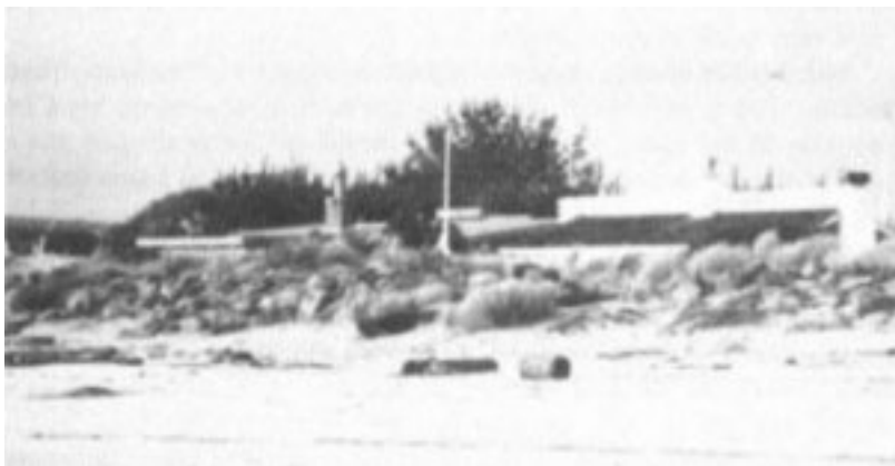
Figure 2-2 Riprap largely covered by accretion of sand, Seadrift, Stinson Beach, California, November 15, 1987. SOURCE: Photo provided by Robert E. Wiegel.
