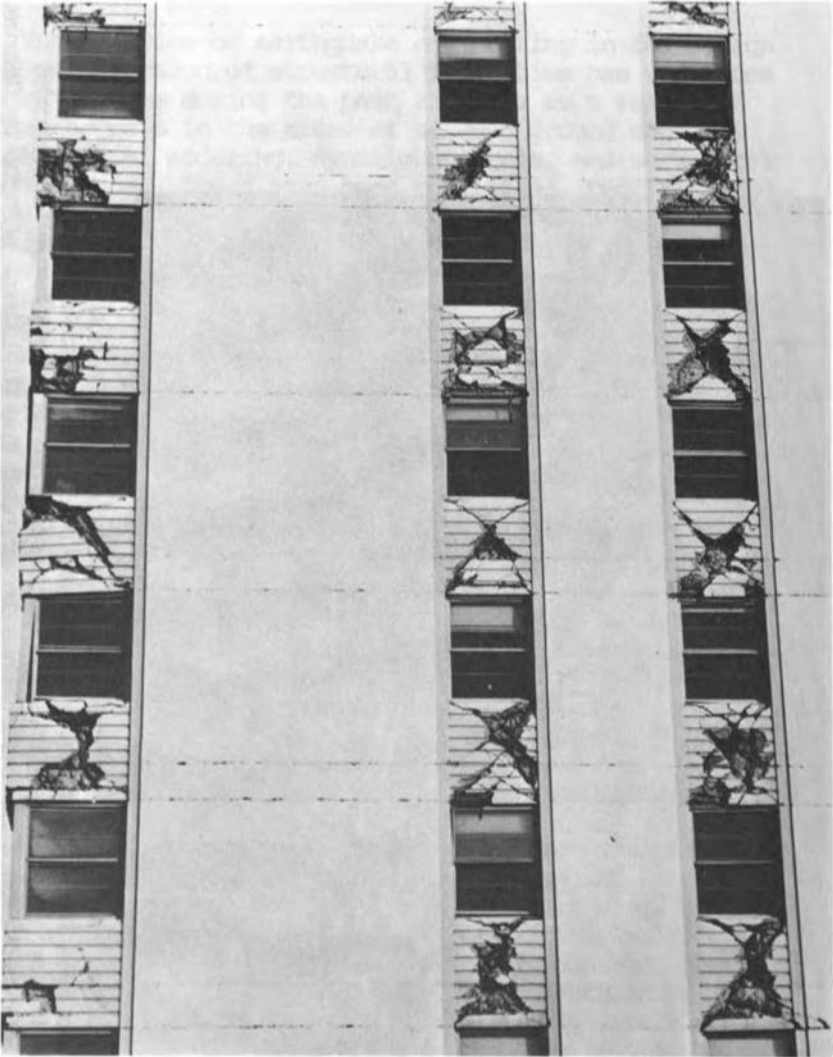
FIGURE 10 This 14-story, reinforced-concrete apartment building in Anchorage, Alaska was damaged by the vibrations produced by the 1964 Alaska earthquake (M8.4). There were no recording instruments in the building, nor were there strong-motion instruments in Alaska at that time. (Photo by George W. Housner)
