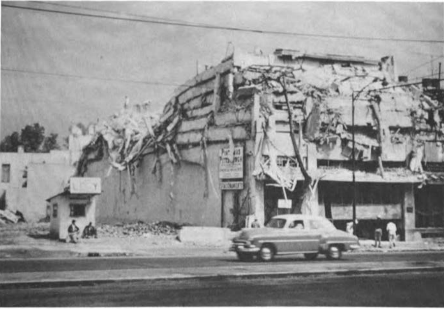
FIGURE 11 Collapse of an eight-story building in Mexico City in 1957. Such collapses, in which the floors are stacked like a deck of cards, have been observed in several earthquakes. The epicenter of the 1957 Mexico earthquake was 200 miles south of Mexico City. Similar collapses occurred during the September 19, 1985 Mexico earthquake. Buildings that were not designed to resist earthquakes are especially susceptible to damage from distant events. (Photo provided by George W. Housner)
