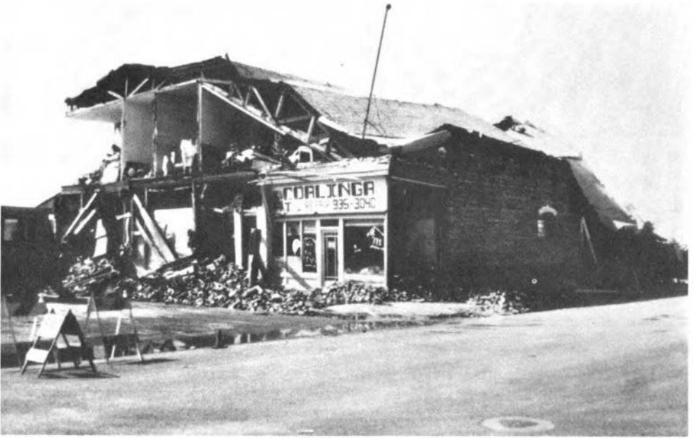
FIGURE 12 Structural damage in the Coalinga business district resulting from the May 2, 1983 earthquake (M6.5). Source: California Division of Mines and Geology (1983). (Photograph by James Stratta)
