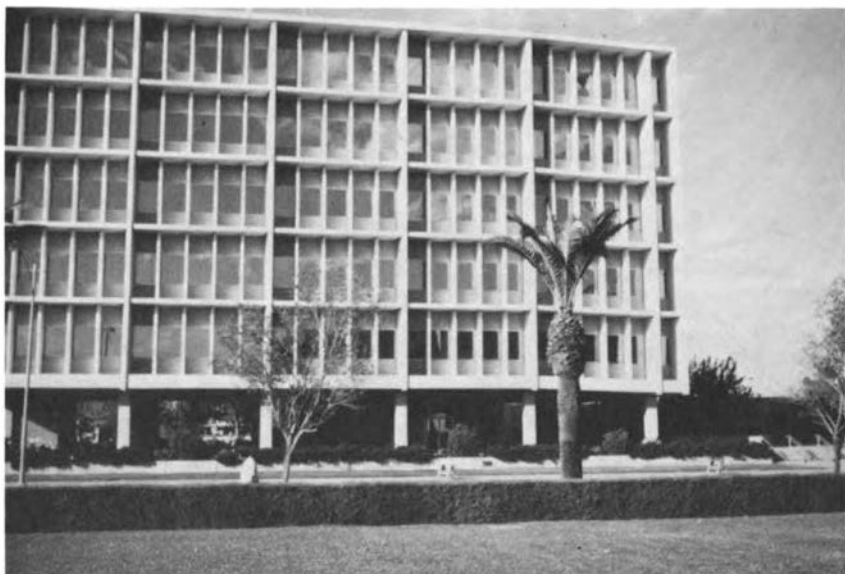
FIGURE 14 View of the south side of the Imperial County Services Building. This structure was severely damaged by the Imperial County earthquake of October 15, 1979 (M6.5). The first-story reinforced-concrete columns were badly cracked at top and bottom. The four columns at the east end of the building were shattered at the bottom and dropped the east end of the building about 10 inches. The building was demolished later. Strong-motion instruments had been installed in the building prior to the earthquake, and these recorded the motions of the roof, several floors, and the ground. Source: California Division of Mines and Geology (1983). (Photo by C. R. Real)
