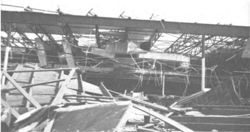
FIGURE 40 Failure of roof in supermarket.
