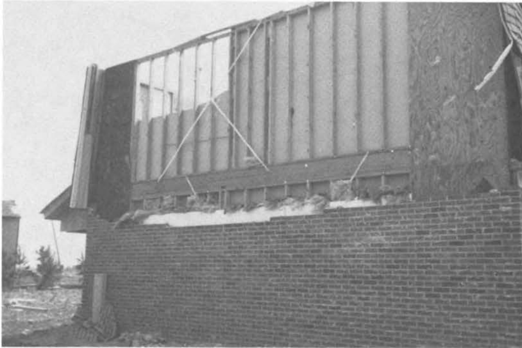
FIGURE 17 Detail of Marlboro Court Apartments showing better bracing.
