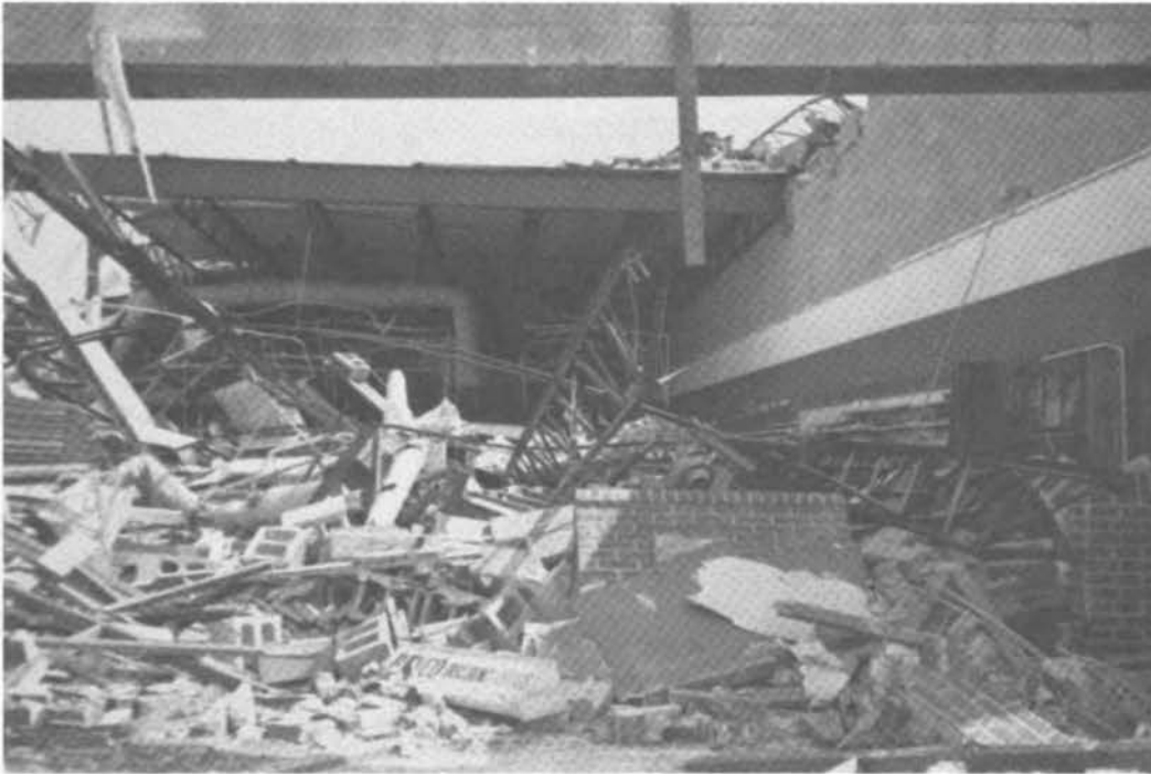
FIGURE 37 Roof collapse in drug store.
