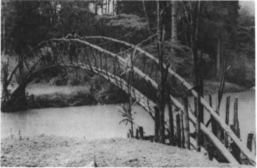
Roundwood. Lagaip River, Papua New Guinea. Flexible young casuarinas joined to form the arch of a bridge. (J. Siegel)
