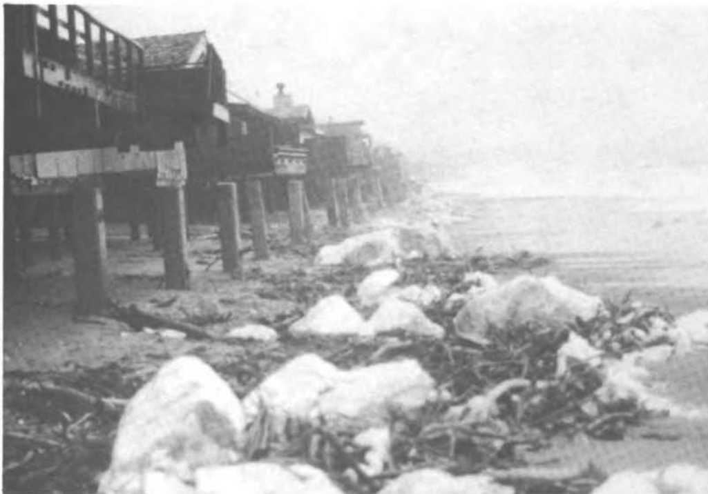
FIGURE 58 Fairly ineffective revetment in Rio Del Mar Beach lowered as a result of scour. The vertical erosion was approximately 2 m.
