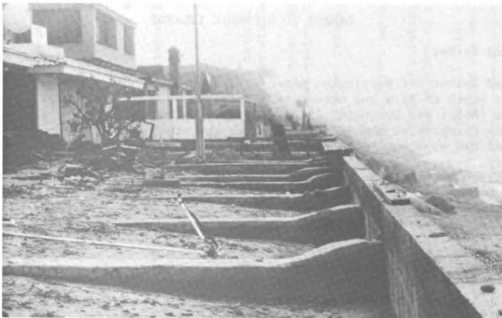
FIGURE 11 Delmar Beach showing the seawall with the damaged Longard tube in the background. Note the effect of the waves overtopping the seawall and causing erosion on the lee side.
