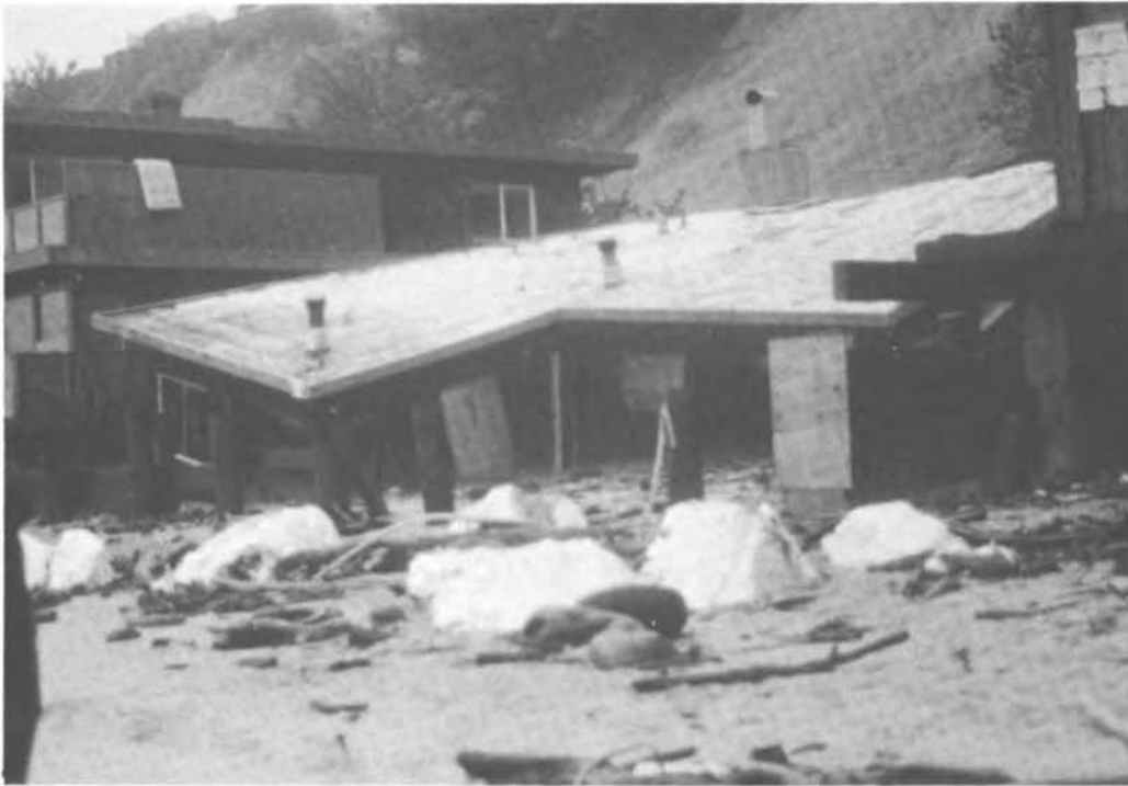
FIGURE 57 Destroyed home in Rio Del Mar Beach with remnants of a poorly designed revetment.
