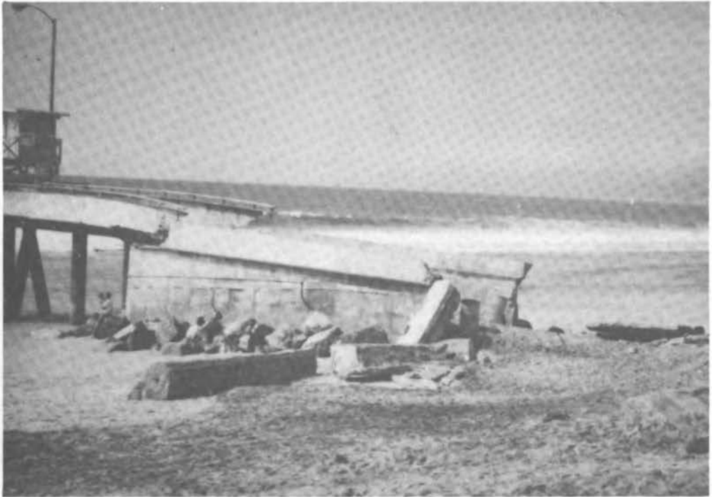
FIGURE 15 The Venice Pier was damaged due to undermining and settlement of the approach ramp.
