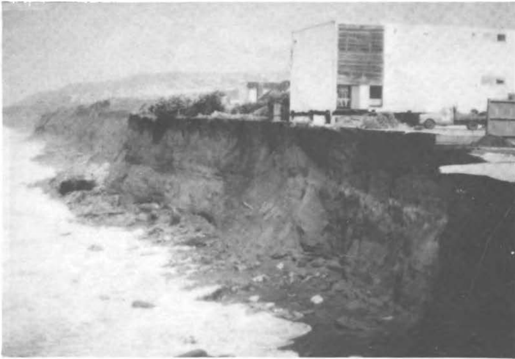
FIGURE 61 Masonic Lodge in Pacifica undercut by wave erosion. The scarp is approximately 10 m high.
