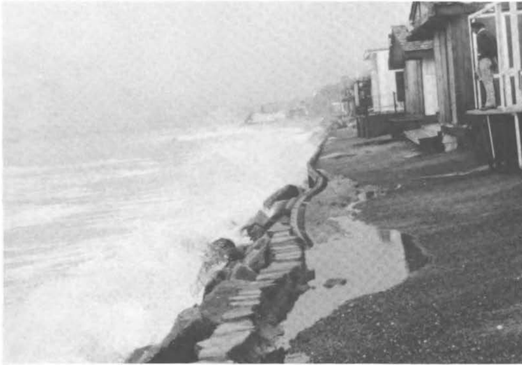
FIGURE 33 Capistrano Shores. A light timber seawall is fronting the trailer park. Note the evidence of overtopping.
