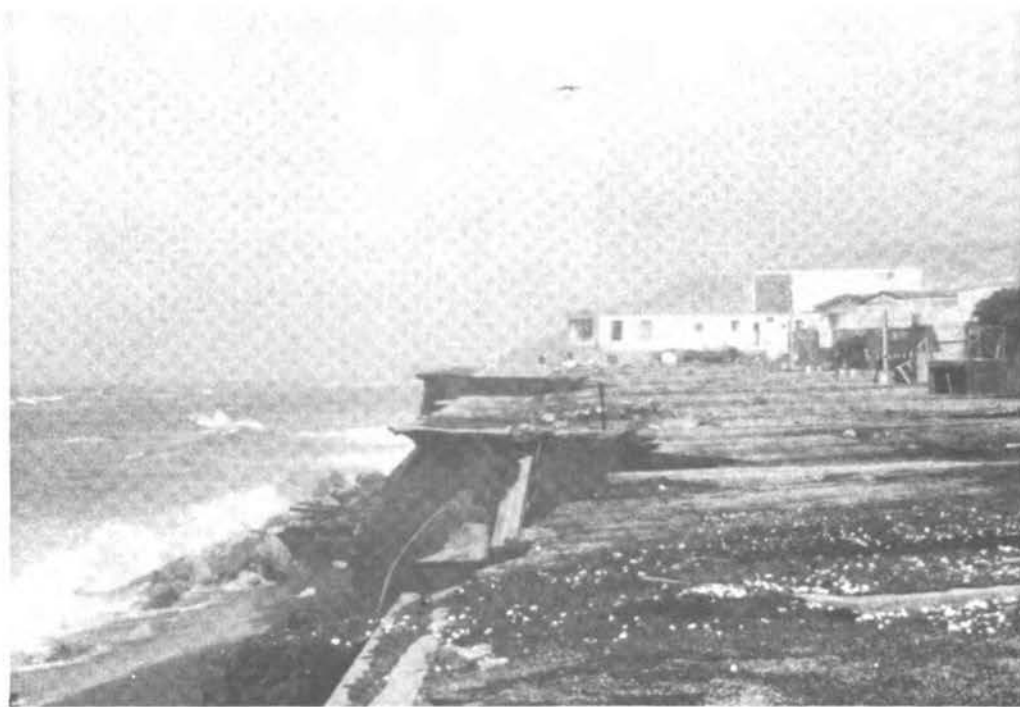
FIGURE 59 Severe erosion in Pacifica adjacent to trailer park.
