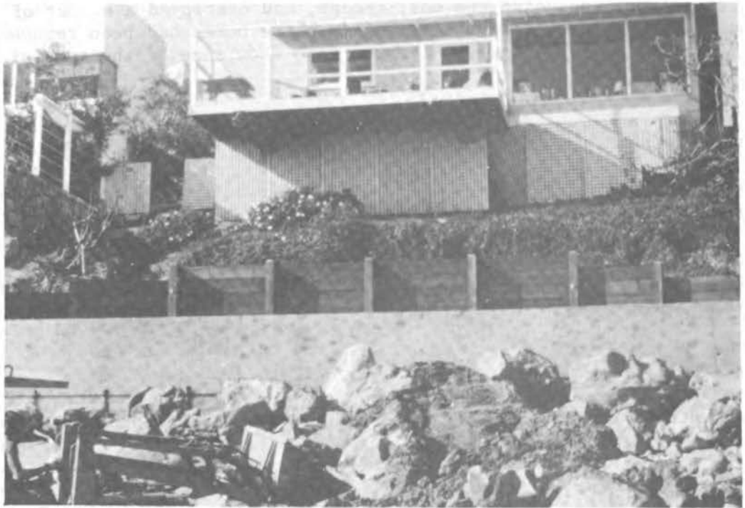
FIGURE 41 Construction during low tide of protective revetment fronting a newly installed seawall.
