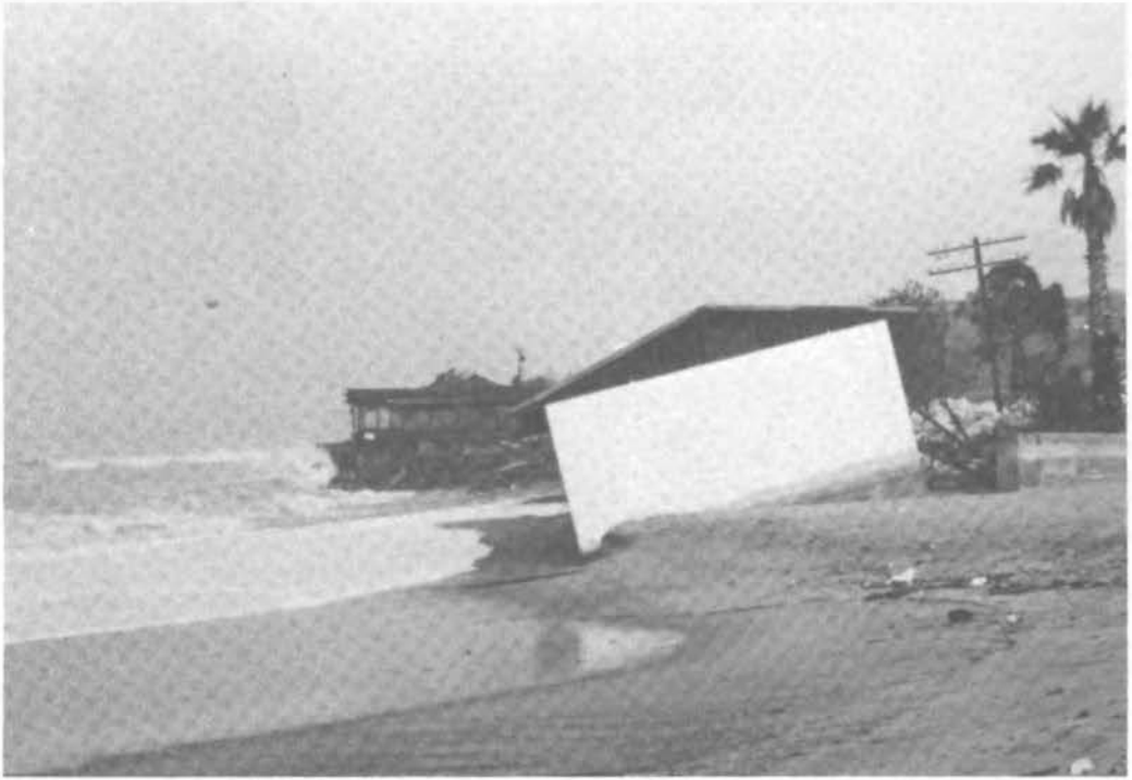
FIGURE 35 This foundation on North San Clemente Beach failed due to undermining of the slab.
