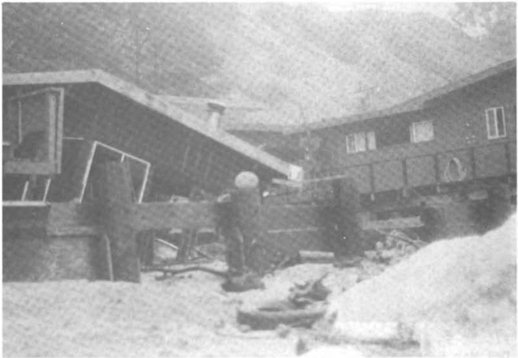
FIGURE 56 Destroyed home in Rio Del Mar Beach fronted by damaged wooden seawall.
