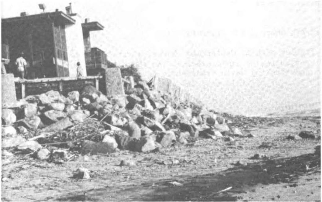
FIGURE 31 Oceanside Beach just south of the mouth of the San Luis Rey River. Heavy revetment and wooden splash guards can be seen. Oceanside Pier is in the background.
