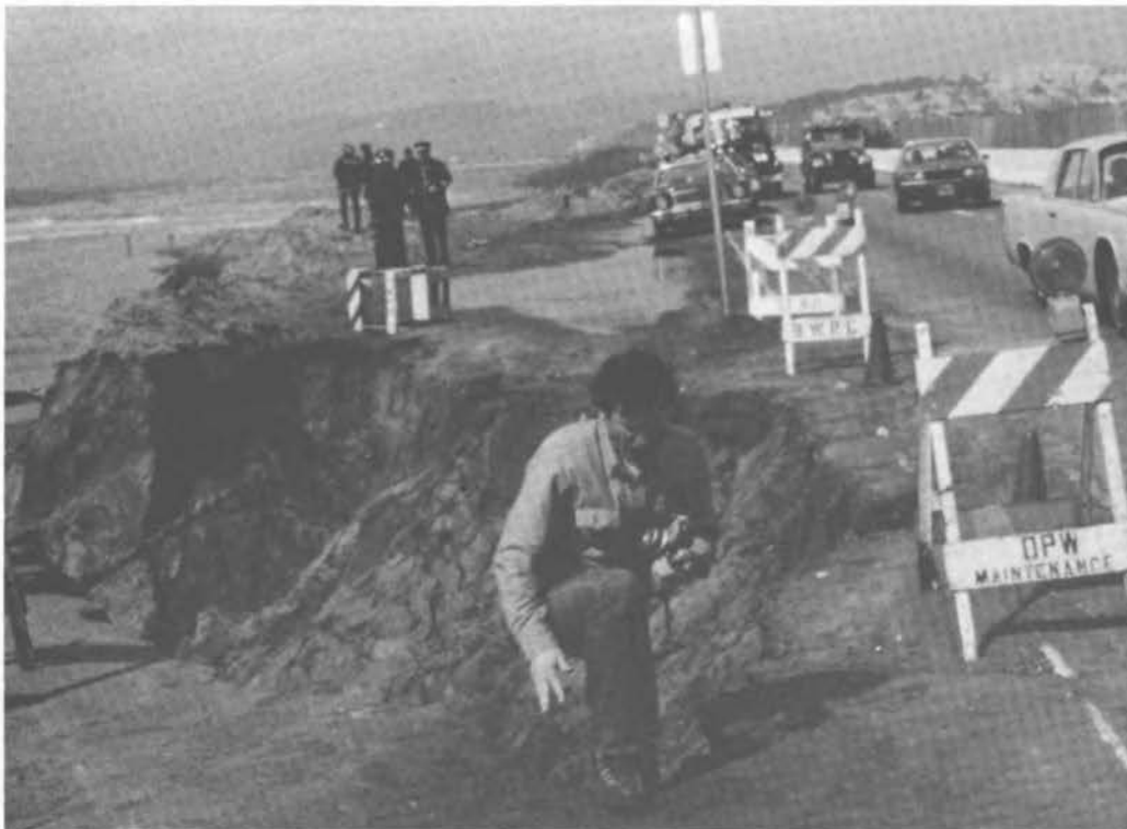
FIGURE 62 Beach erosion and road damage at Ocean Beach south of the entrance to San Francisco Bay.
