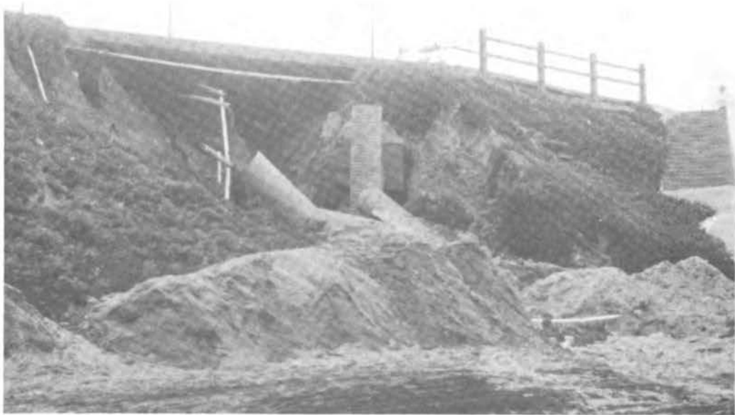
FIGURE 40 Torrance County Park. This view toward land shows damage to drainage conduits and water lines. The erosion was probably due to a combination of waves and runoff.
