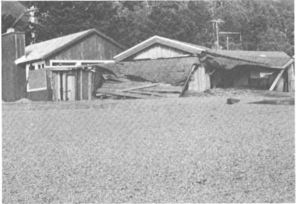
FIGURE 67 Structures in Stinson Beach damaged and destroyed from erosion undermining and direct action of waves.
