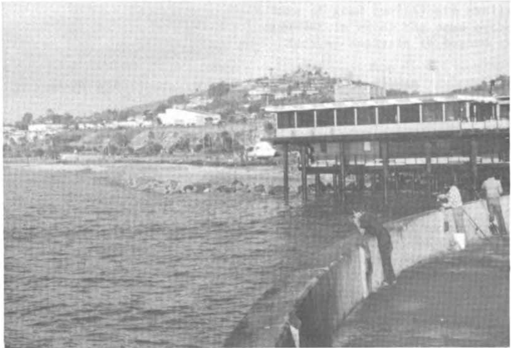
FIGURE 9 Revetment adjacent to the Santa Barbara Yacht Clubhouse at the base of the Santa Barbara breakwater. Note the complete loss of sand from behind the revetment.
