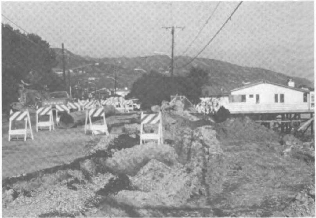
FIGURE 45 Road damage in Malibu Beach due to wave or runoff erosion.
