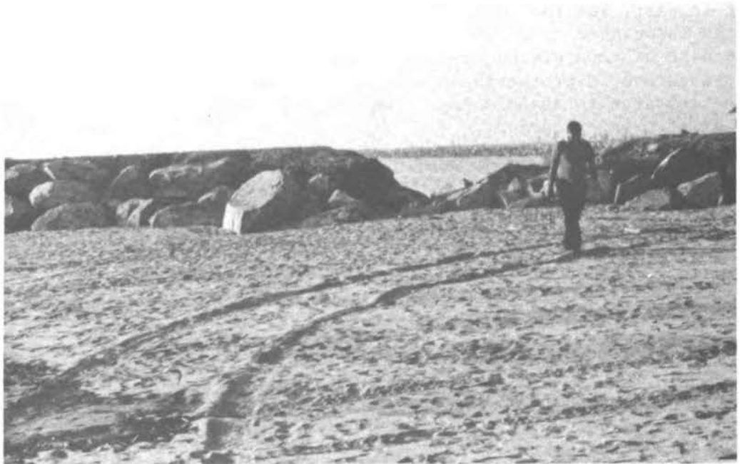
FIGURE 32 Small breach in the south breakwater at Oceanside Harbor.
