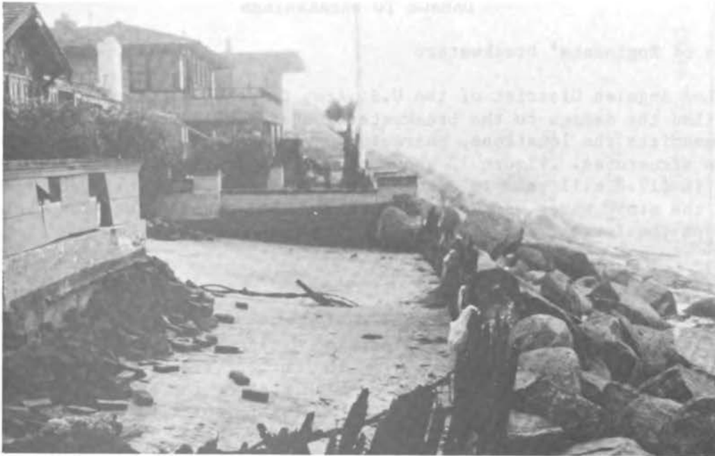
FIGURE 10 A view of Delmar Beach showing the light ineffective seawall, revetment, and damaged Longard tube. Note the small Caterpillar in the background moving sand to the upper portions of the beach.
